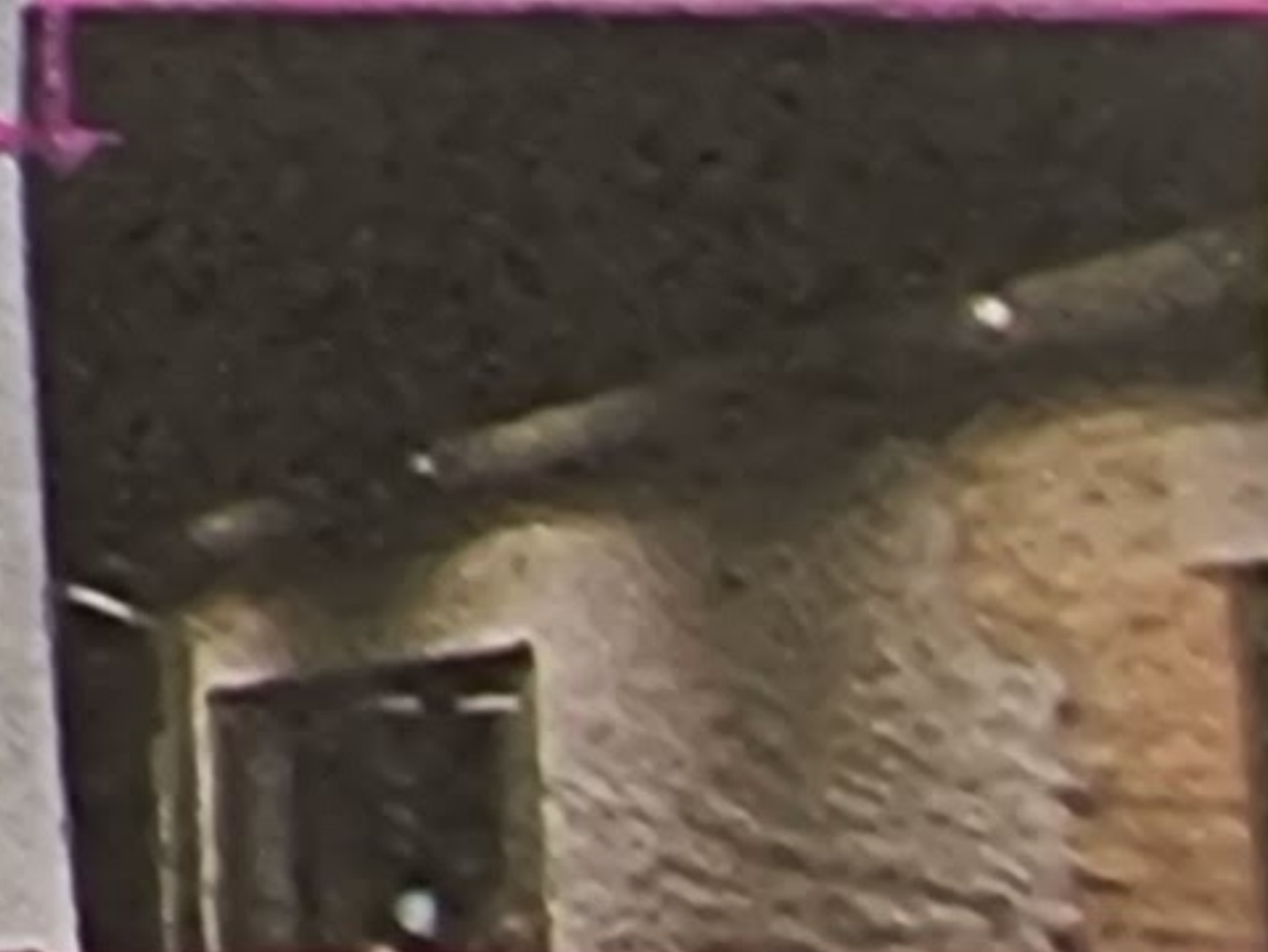
LED Down Lights – Downward facing spots lights used to light under ground floor overhang
