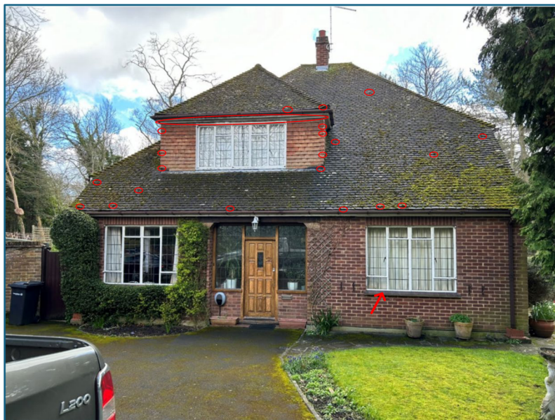
Figure 5: PRFs visible on the western facing elevation
