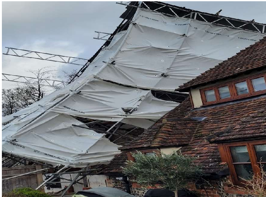
Scaffold Collapse Rear
