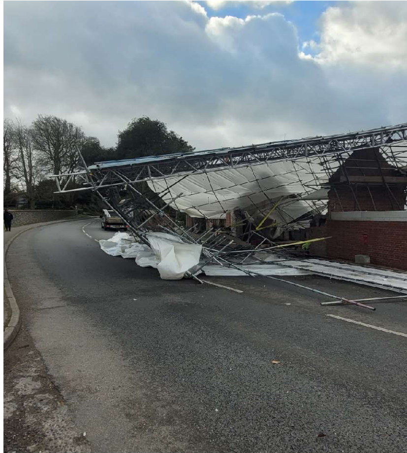
Scaffold Collapse Front
