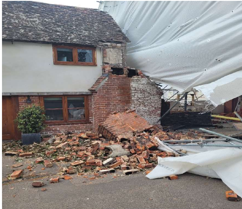
Front Chimney Damage
