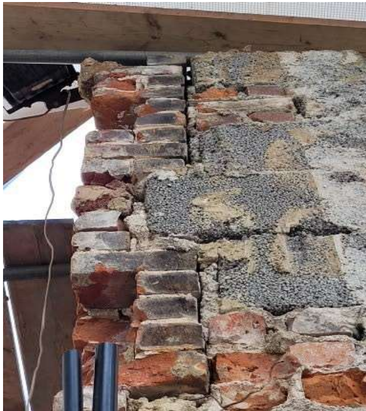
Gable End Wall Damage
