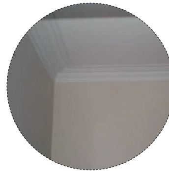
Neighbouring property application evidence of matching cornice to that on site
