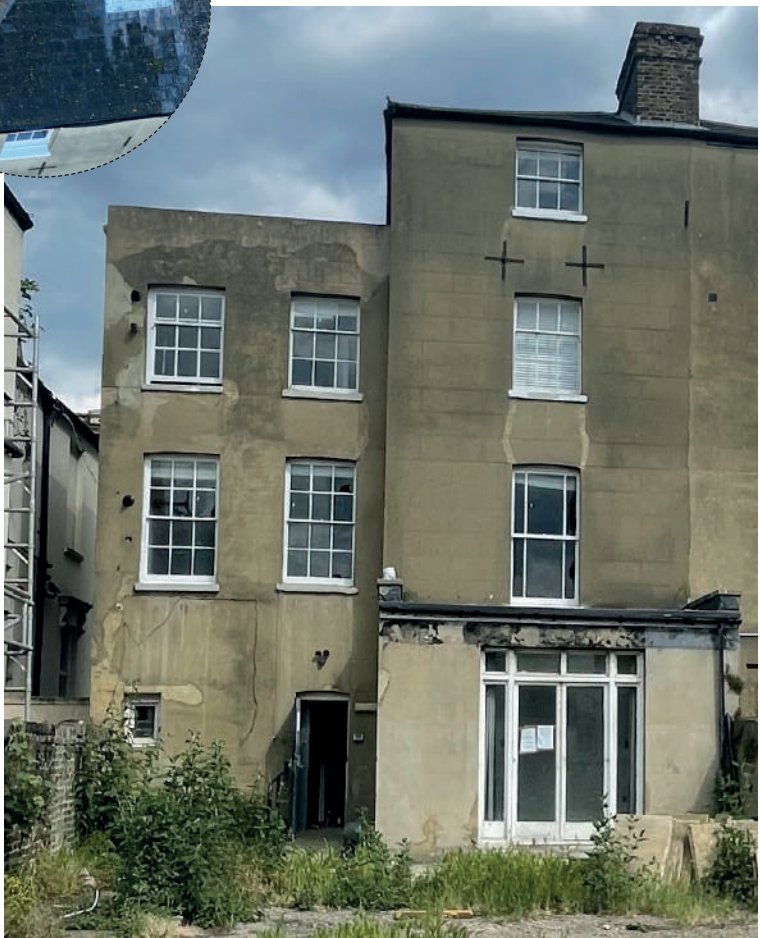
Fig 18 Site photo Rear Elevation by JCA Oct 2025: Evidencing no external works having been carried out
