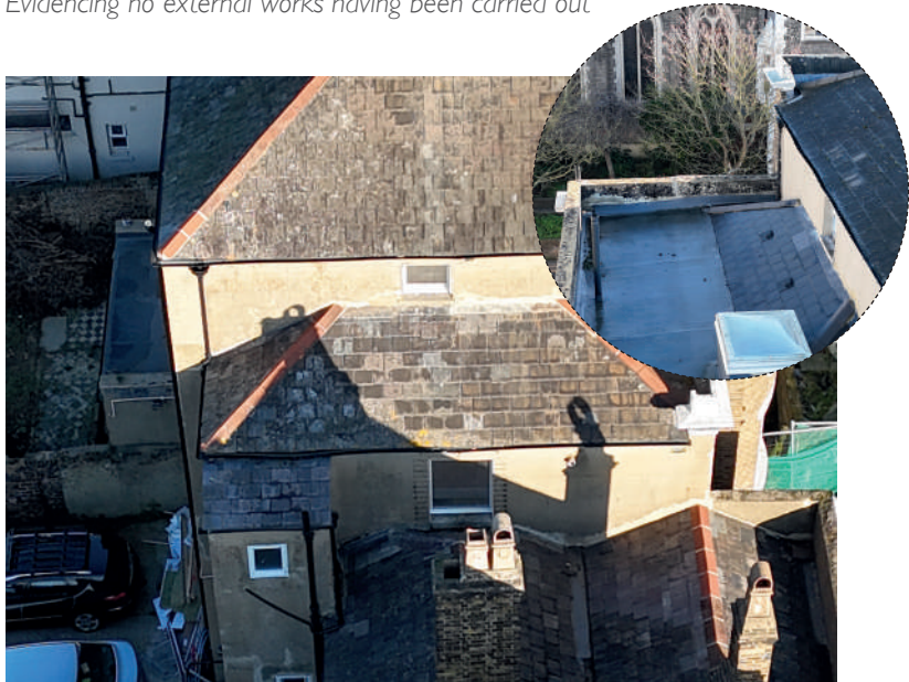
Fig 19 Left: Site photo by JCA Oct 2025: Evidence of aborted work and temporary structural measures to Lower Ground Floor bay;; Fig 14b (callout) light-well wall upstand construction; 14c right: Drone footage by JCA Oct 2025: Evidencing original hipped slate roof wing of no. 196 to which it is assumed no. 195 mirrored prior to the additional flat roof extension; 14d (callout) No. 195 slate roof remains, AOV inserted within)
