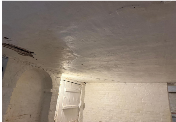
Photograph 1: Existing water-damaged lath and plaster ceiling.
