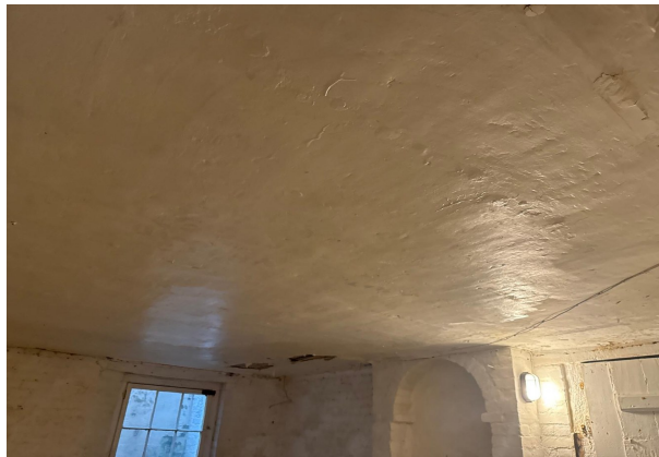
Photograph 3: Existing water-damaged lath and plaster ceiling.
