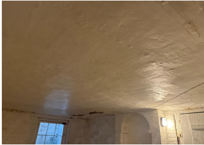
Photograph 3: Existing condition of the water-damaged lath and plaster ceiling at Jeskyns Court. Photographs show areas of cracking, plaster loss and exposed laths.
