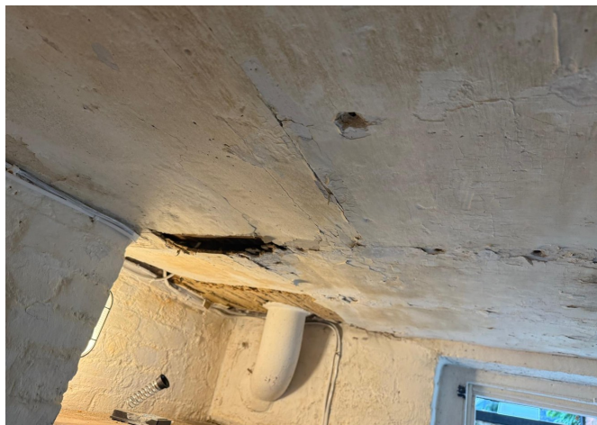
Photograph 8: Existing condition of the water-damaged lath and plaster ceiling at Jeskyns Court. Photographs show areas of cracking, plaster loss and exposed laths.
