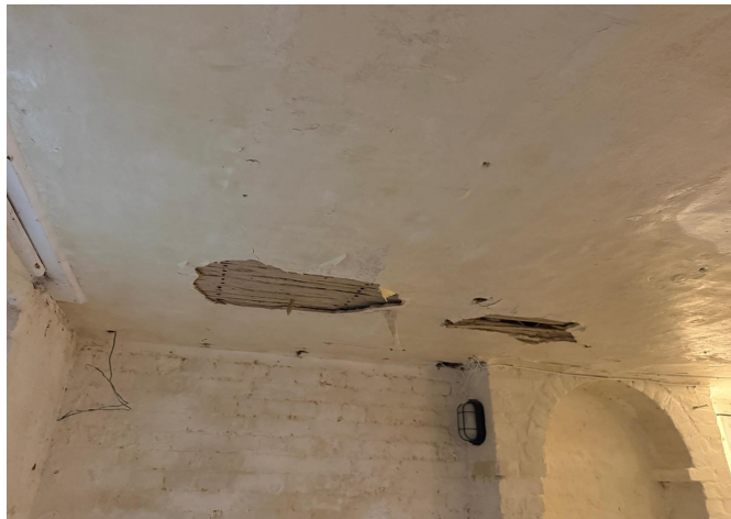
Photograph 10: Existing condition of the water-damaged lath and plaster ceiling at Jeskyns Court. Photographs show areas of cracking, plaster loss and exposed laths.
