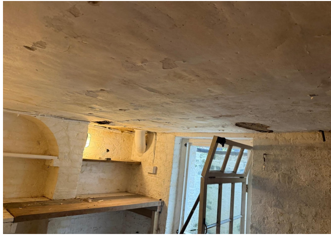
Photograph 9: Existing condition of the water-damaged lath and plaster ceiling at Jeskyns Court. Photographs show areas of cracking, plaster loss and exposed laths.
