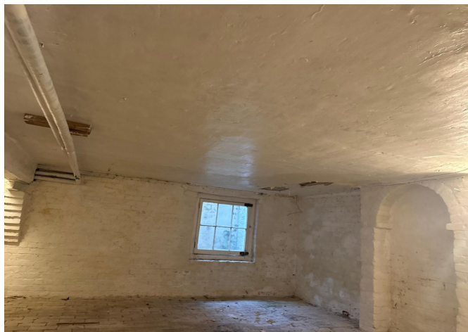
Photograph 5: Existing condition of the water-damaged lath and plaster ceiling at Jeskyns Court. Photographs show areas of cracking, plaster loss and exposed laths.
