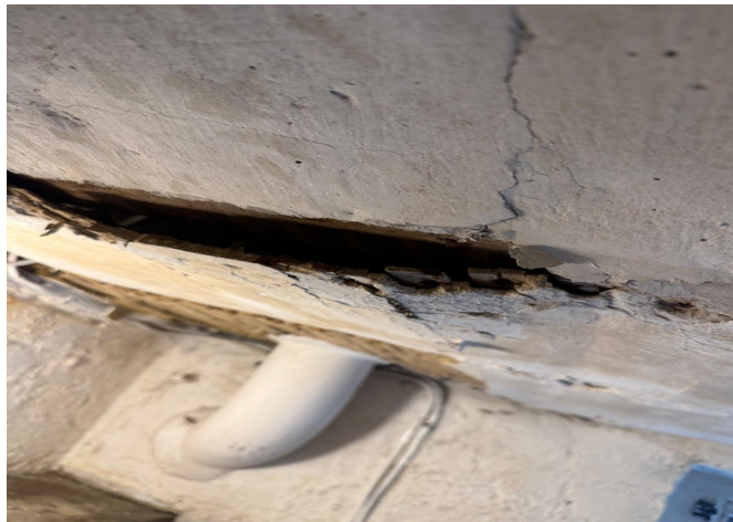
Photograph 7: Existing condition of the water-damaged lath and plaster ceiling at Jeskyns Court. Photographs show areas of cracking, plaster loss and exposed laths.
