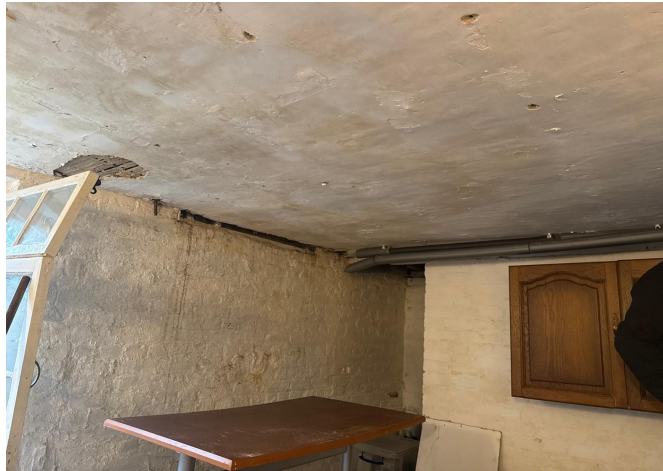
Photograph 6: Existing condition of the water-damaged lath and plaster ceiling at Jeskyns Court. Photographs show areas of cracking, plaster loss and exposed laths.
