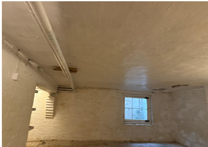
Photograph 4: Existing condition of the water-damaged lath and plaster ceiling at Jeskyns Court. Photographs show areas of cracking, plaster loss and exposed laths.
