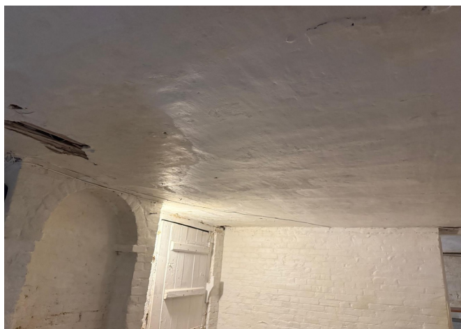
Photograph 1: Existing condition of the water-damaged lath and plaster ceiling at Jeskyns Court. Photographs show areas of cracking, plaster loss and exposed laths.
