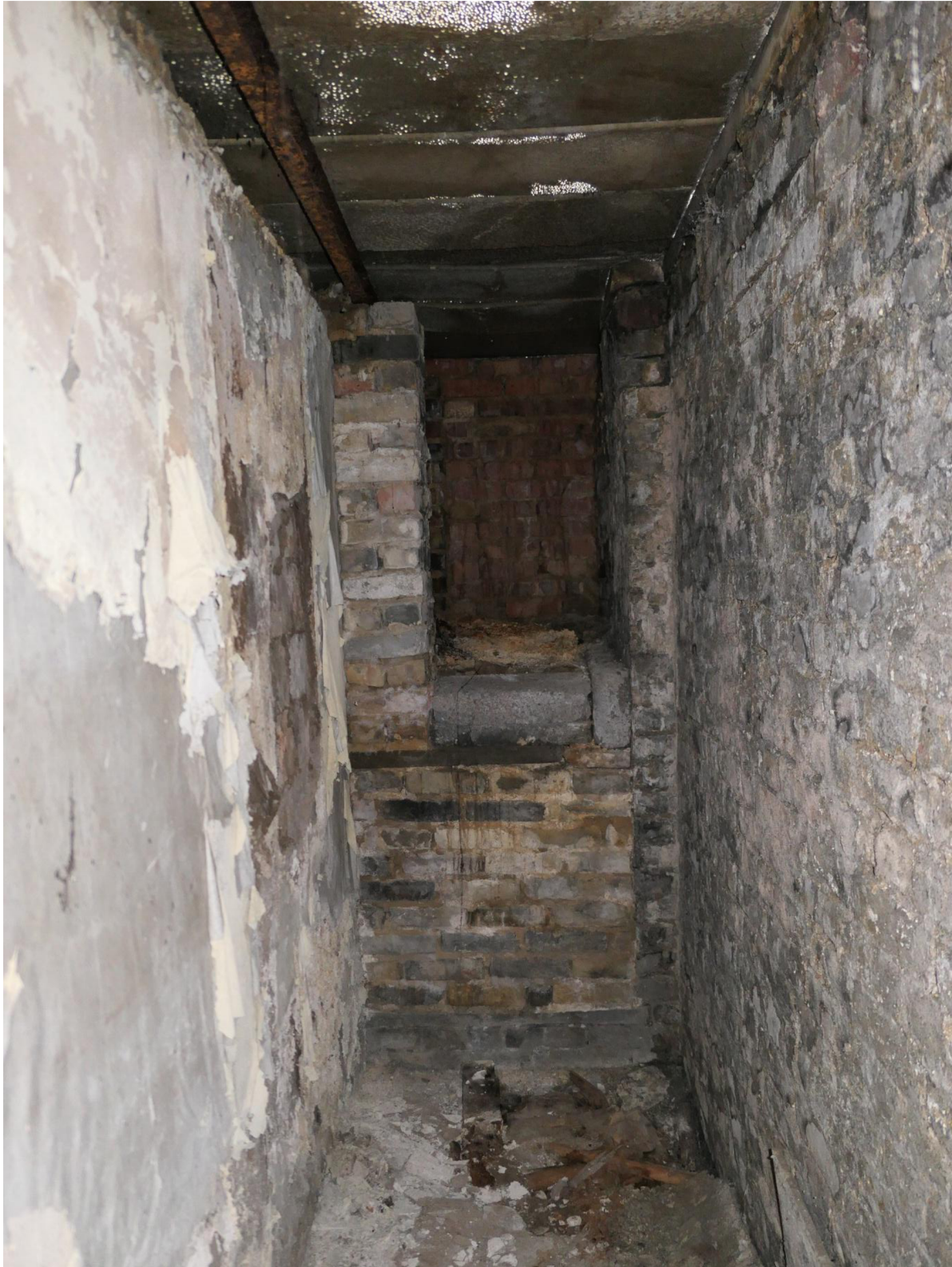
Photo 6: the front basement light well has been covered, but survives in a fossilised way, with the front basement window filled with blockwork.
