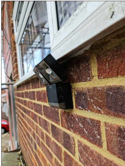
EXISTING TWIN MOTION SENSOR FLOOD LIGHT
