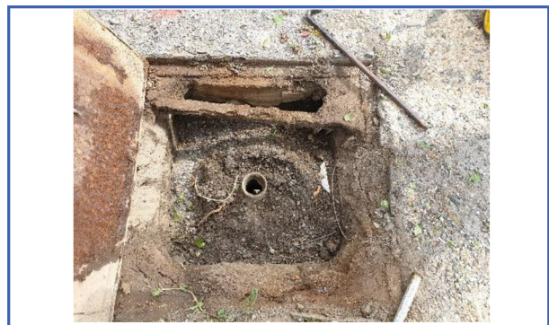
Fill point infrastructure within manhole
