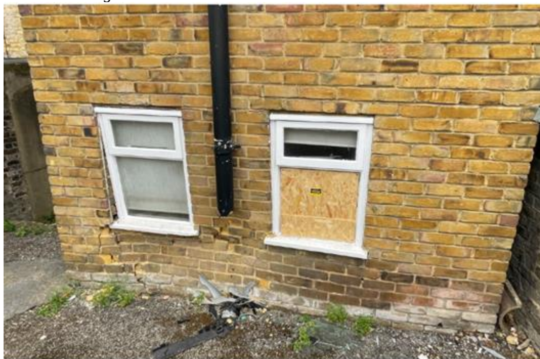
Photo of Damage
