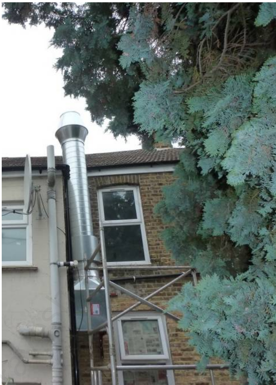
Photo of Extractor installed to rear of the property
