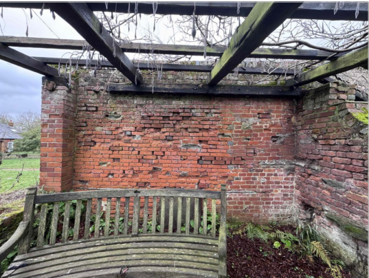
1. VIEW SHOWING CONDITION OF BRICK SPINE WALL
