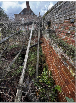
4. VIEW OF SPINE WALL AND COLLAPSED TIMBER STRUCTURE FROM ABOVE
