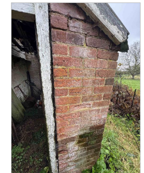
5. SOUTH EAST BRICK WALL - SHOWING DAMP
