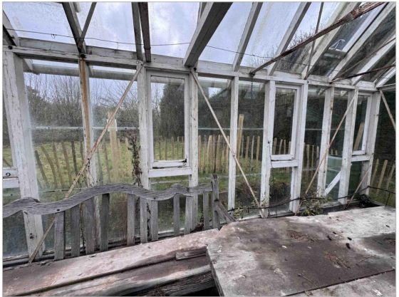
5. INTERNAL VIEW SHOWING CONDITION OF TIMBER WINDOWS
