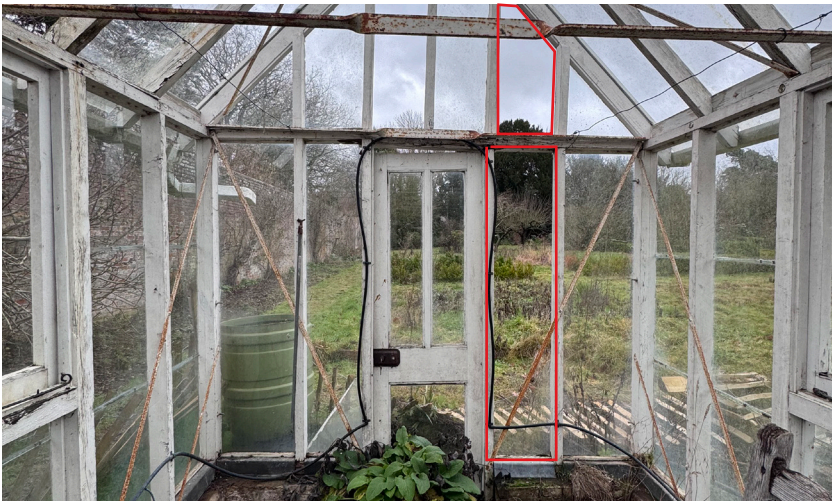
4. Internal view - showing broken glass panes highlighted in red
