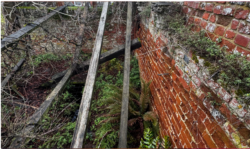
7. View of Loggia showing collapsed timber structure from above
