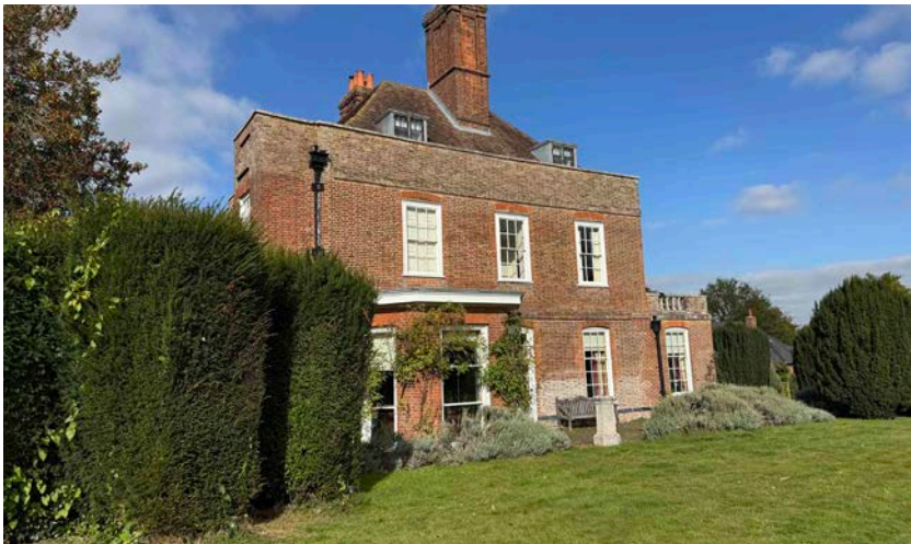
1. South-eastern elevation showing affected gutter outlet
