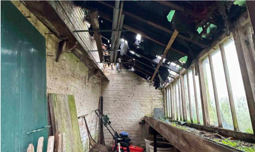
3. Internal photo showing decayed timber structure and failing tarpaulin
