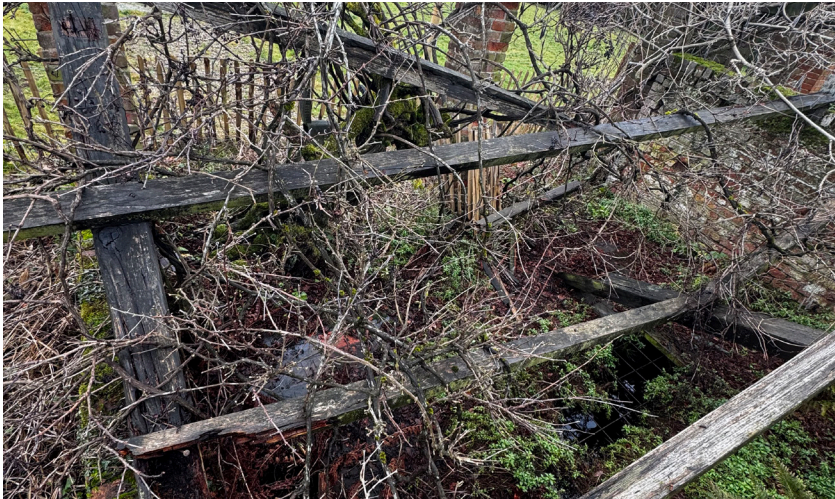
5. View of Loggia from above showing timber roof collapse
