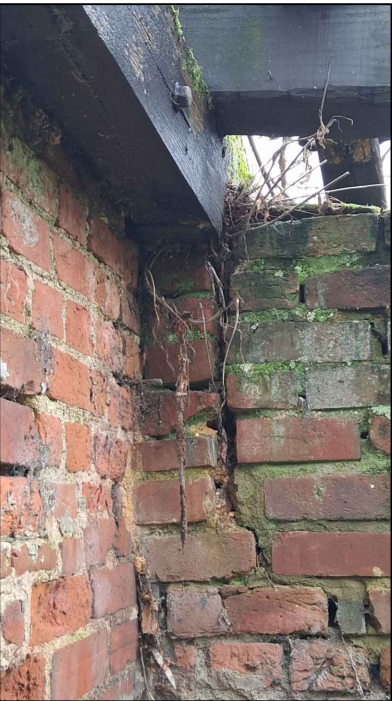
PHOTO 1 - CRACK IN BRICKWORK UNDERNEATH TIMBER WALL PLATE
