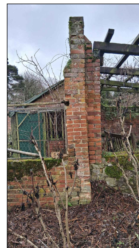
PHOTO 2 - CRACK IN BRICKWORK NEAR BOTTOM OF BRICK WALL
