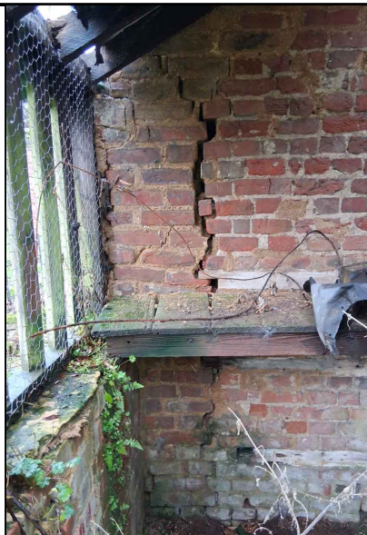
PHOTO 3 - 15 mm WIDE VERTICAL CRACK ALL THE WAY TO GROUND LEVEL.
