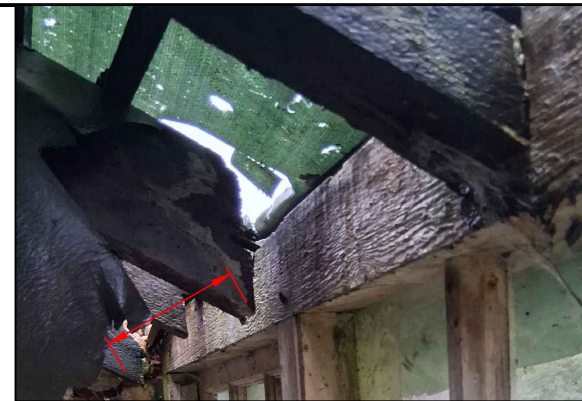
PHOTO 5 - 3 NO. RAFTER ENDS NOT BEARING ONTO STUD WALL AT EAVES LEVEL.
