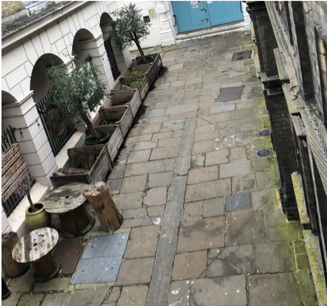
Figure 9 Replace/Re bed damaged/undulated pavers within thoroughfare
