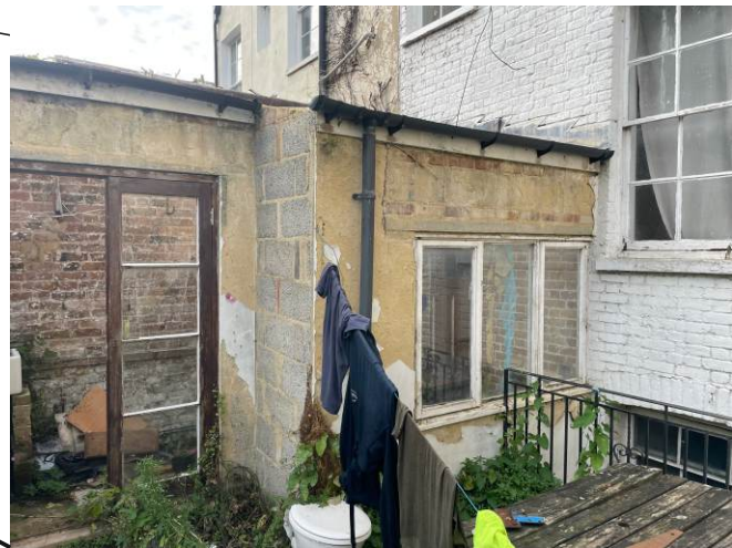
PHOTOGRAPH 2 Showing extension at first floor it can be seen it is poor condition with a collapsed roof. The walls are single skin rendered block work and non - original. It also shows that existing facing brickwork to the rear has been painted white.
