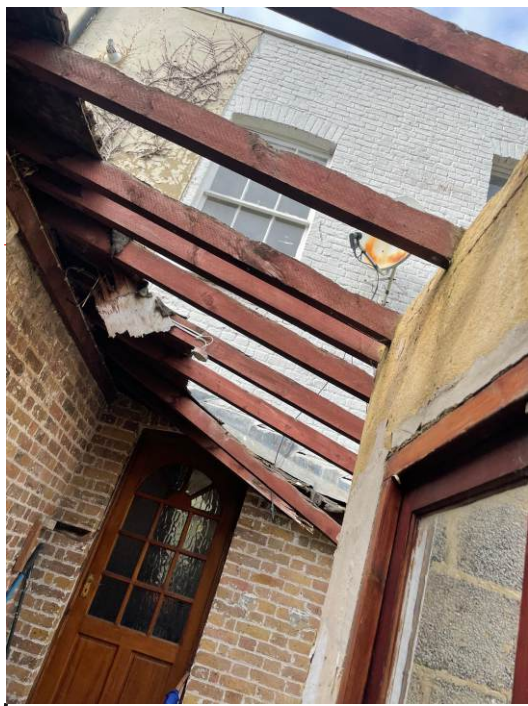
PHOTOGRAPH 7. Showing derelict rear addition
