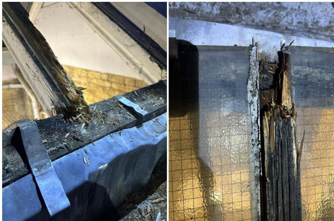
Figure 5: Rotten timber glazing bars of platform 2 canopy
