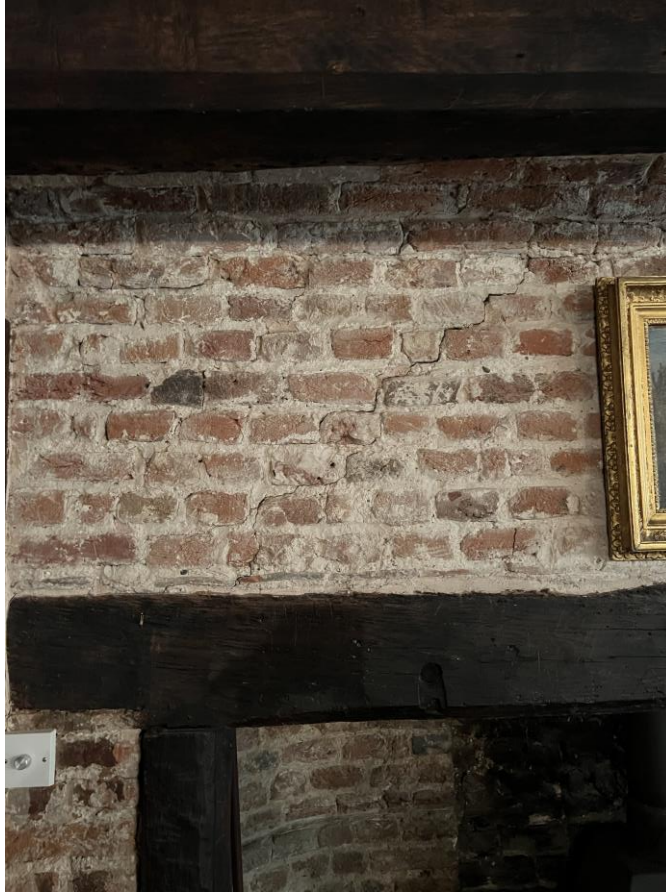
Image of the crack above the bressummer in the ground floor of the axial chimney facing west.
