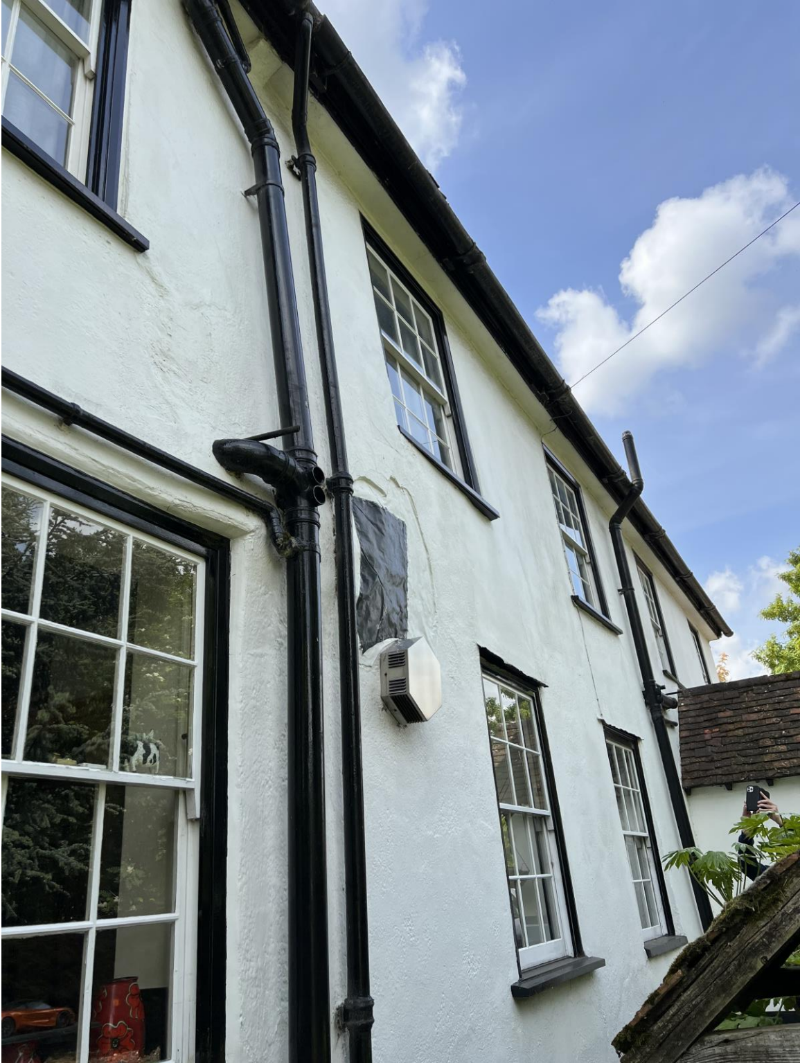
Bulge in external render on north elevation
