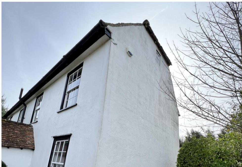
Roof verges do not extend fully beyond the face of the rendered wall.
