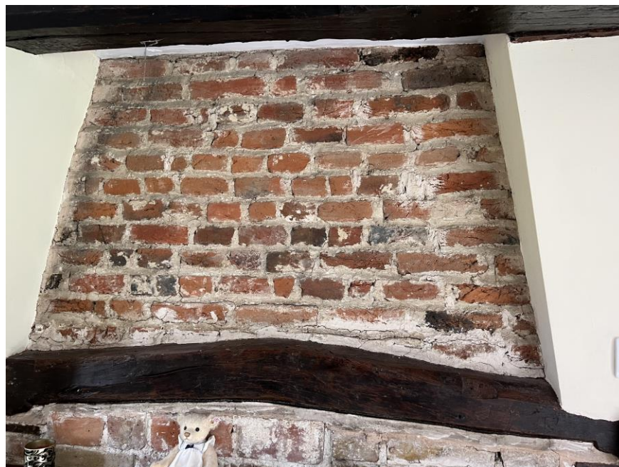
Image of the cracking above the bressummer in the first floor of the axial chimney facing west.
