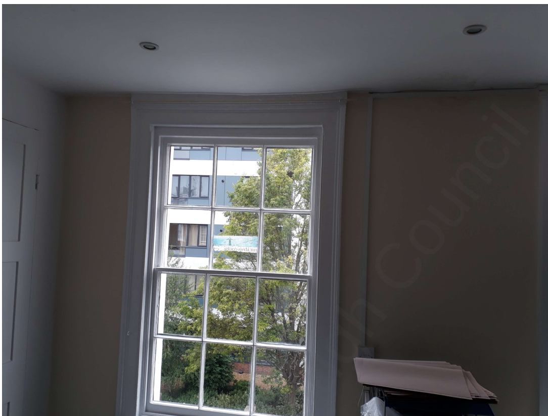
No.57's second floor front window demonstrating there is no cornice detail.
