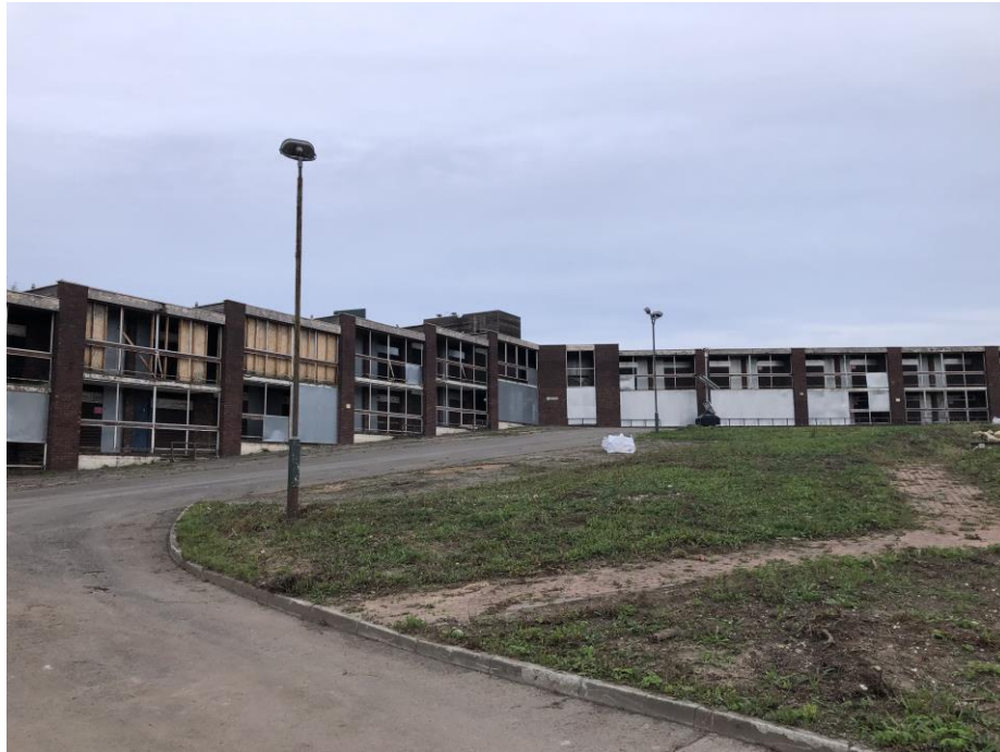
VP3 hotel accommodation building with column mounted floodlighting to illuminate courtyard and service road.
