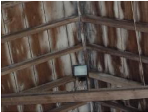
1. Image above shows the underside of the ridge, with some staining to the timbers. The extent of any decay or damage cannot be assessed until work commences. All repairs will be carried out on a like for like basis using the same materials as existing.
