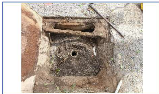
Fill point infrastructure within manhole
