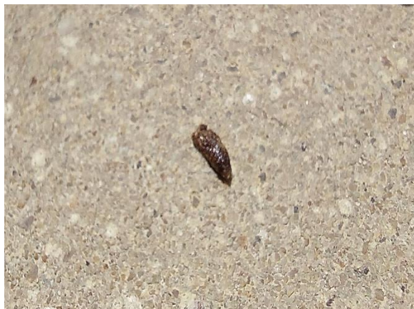
Dropping found on the east elevation of building B9.
