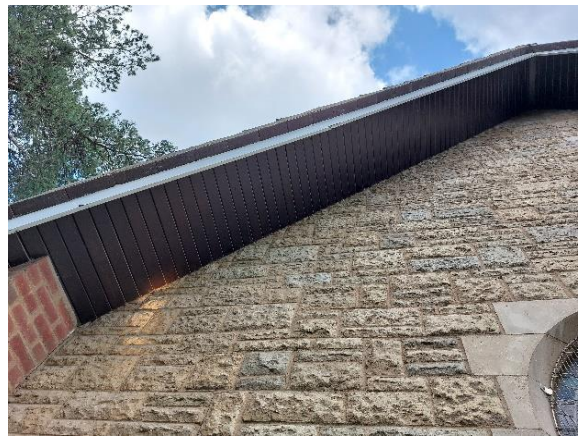
Gaps under the soffit of building B9 (east elevation).
