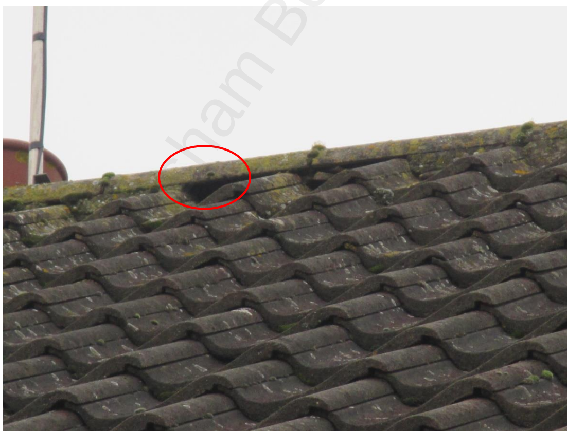
Photograph 2 – PRFs are present on the ridgeline where mortar is missing.
