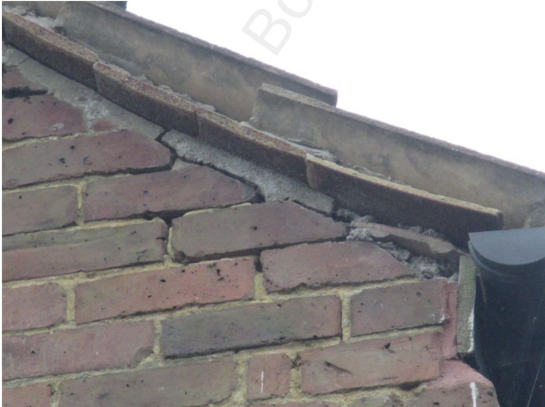
Photograph 6 – Cavities are present in the mortar beneath the end roof tiles on the northern gable end, however these are superficial and considered to be unsuitable for roosting bats.
