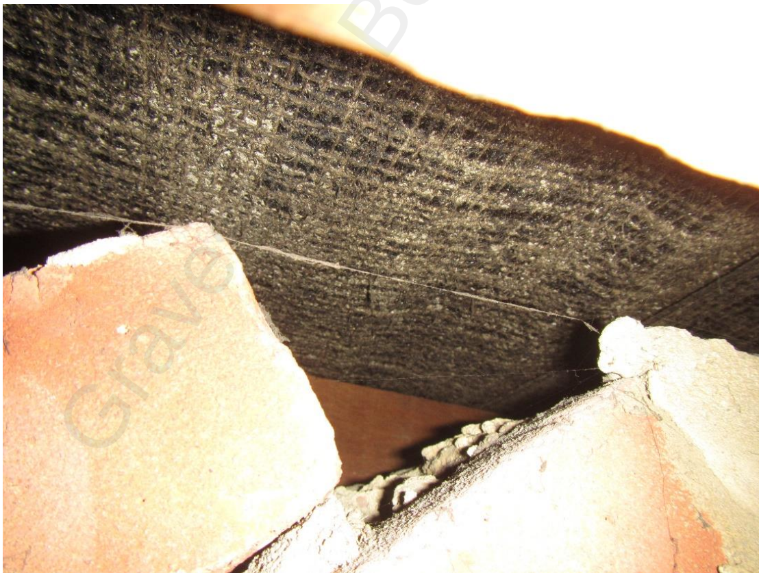
Photograph 10 – Cavity present at the edge of the wall at the southern end of the loft void.
