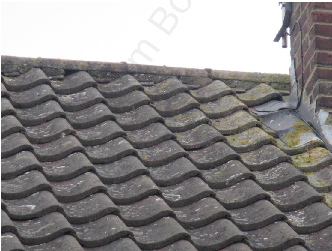
Photograph 4 – The central redbrick chimney is in good condition, however PRFs are present beneath the raised lead flasing.
