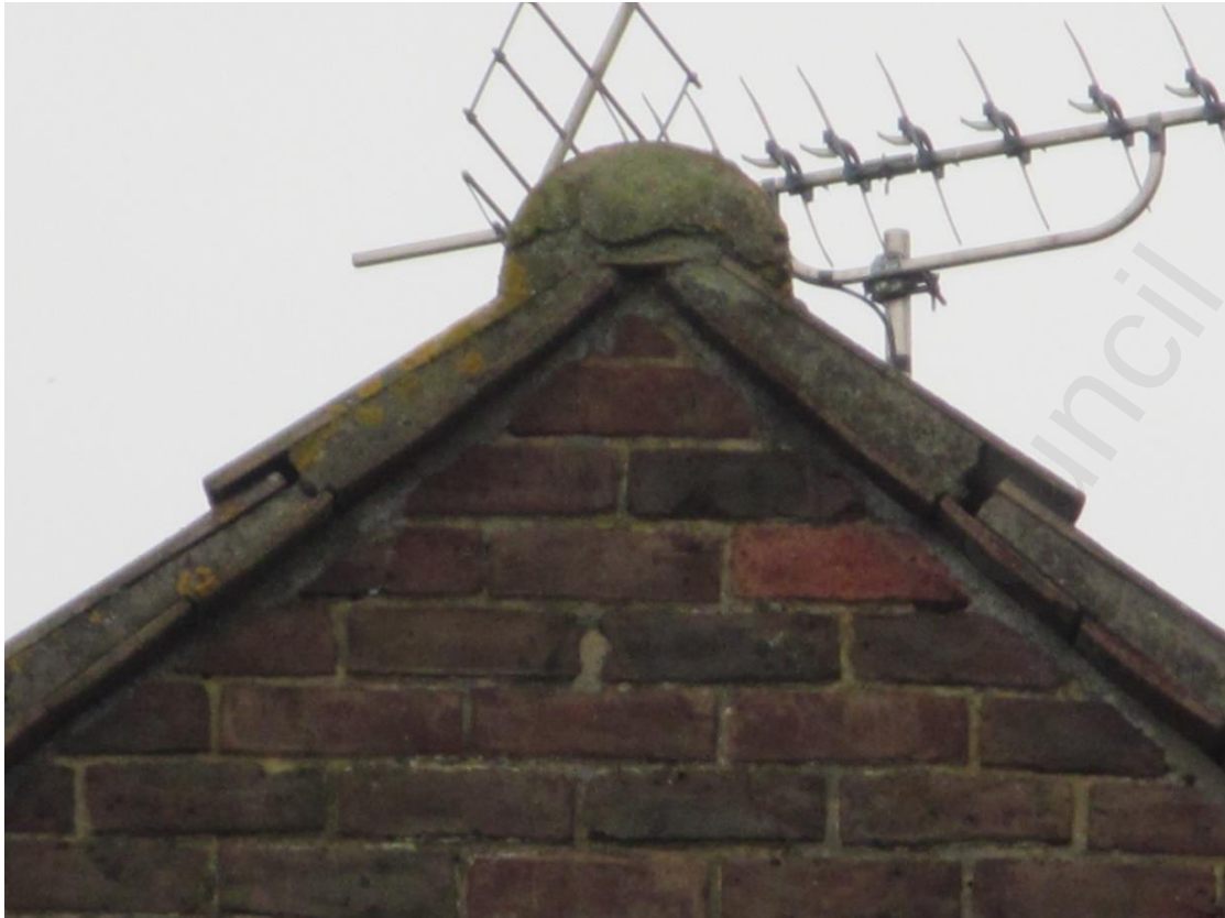
Photograph 5 – PRFs are present where the mortar is missing between end tiles at the northern gable end of the building.
