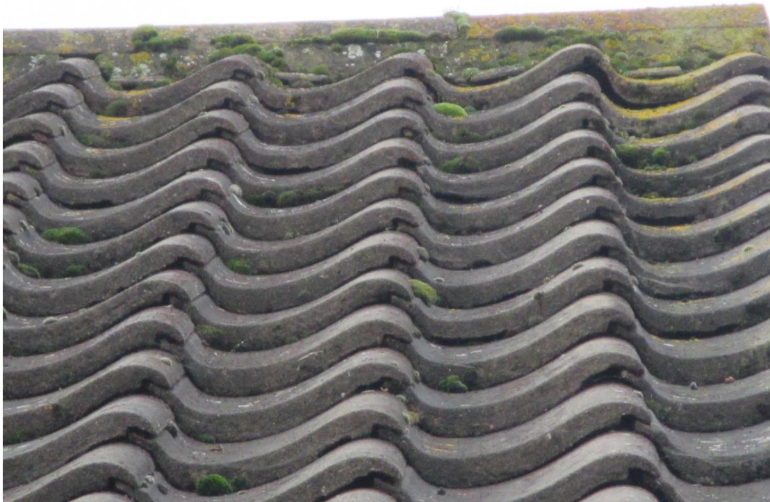
Photograph 3 – Numerous PRFs are present beneath raised roof tiles.
