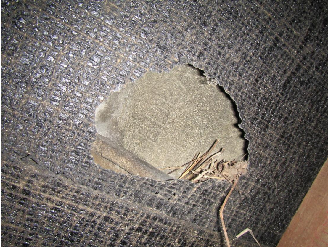
Photograph 11 – A historical bird nest (suspected to have been house sparrow) was observed within a tear in the bitumen membrane, located between the membrane and the roof tiles.
