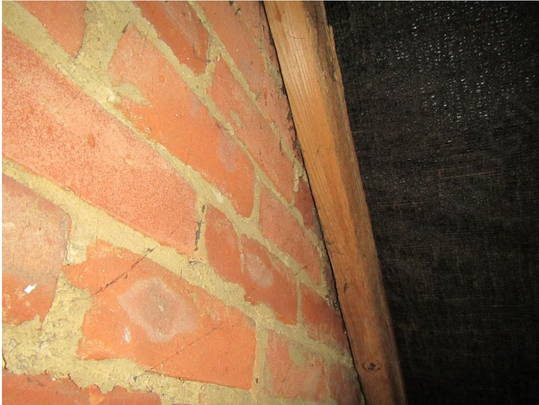
Photograph 9 – Cavities are present between the end rafter and the brick wall at the northern end of the loft void.
