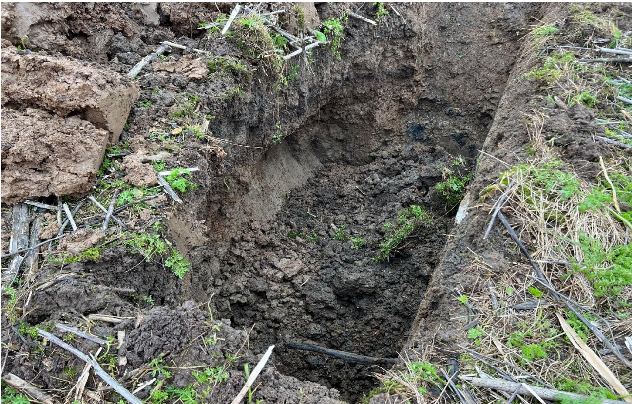
TP-13 Collapsed (no face pics)
