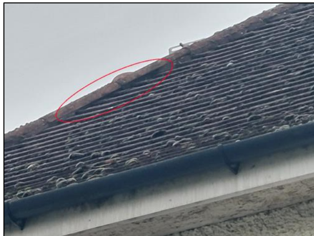
Photograph 2. Missing pugging from below the ridge tile on the left side of the rear elevation as highlighted in red.
