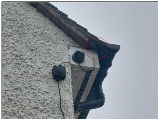
Photograph 4. Gap present where tile does not meet the timber frame on the right side of the rear elevation as highlighted in red.
