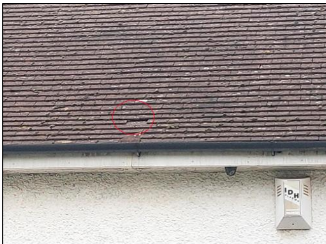
Photograph 3. Missing tile from the roof on the left side of the rear elevation as highlighted in red.
