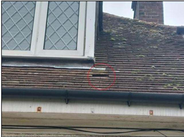
Photograph 7. Missing tile from the roof on the right side of the front elevation as highlighted in red, feature discounted as the stub of tile can be seen with binoculars.
