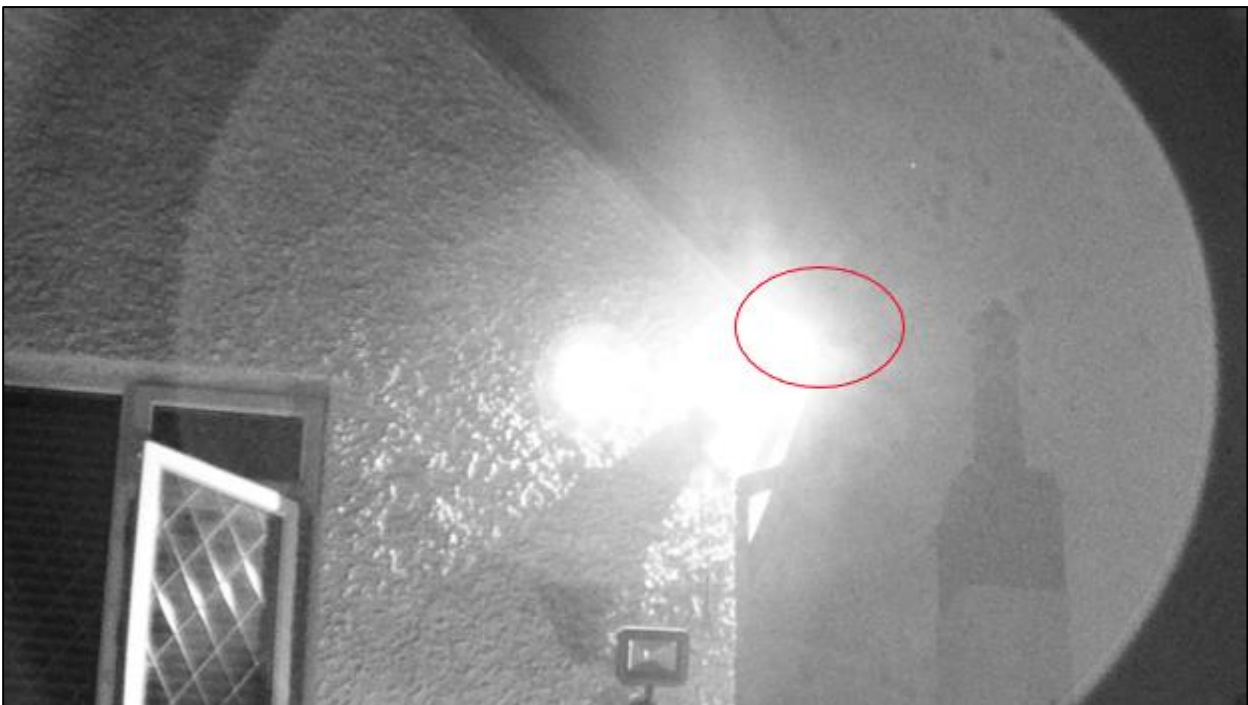
Figure 3. The darkest point from the camera facing the eastern elevation, gap where soffit box does not meet the timber frame (highlighted with red circle). This feature was obstructed by the exterior lighting for the camera, however the surveyor did not note any emergences from this location during the survey.
