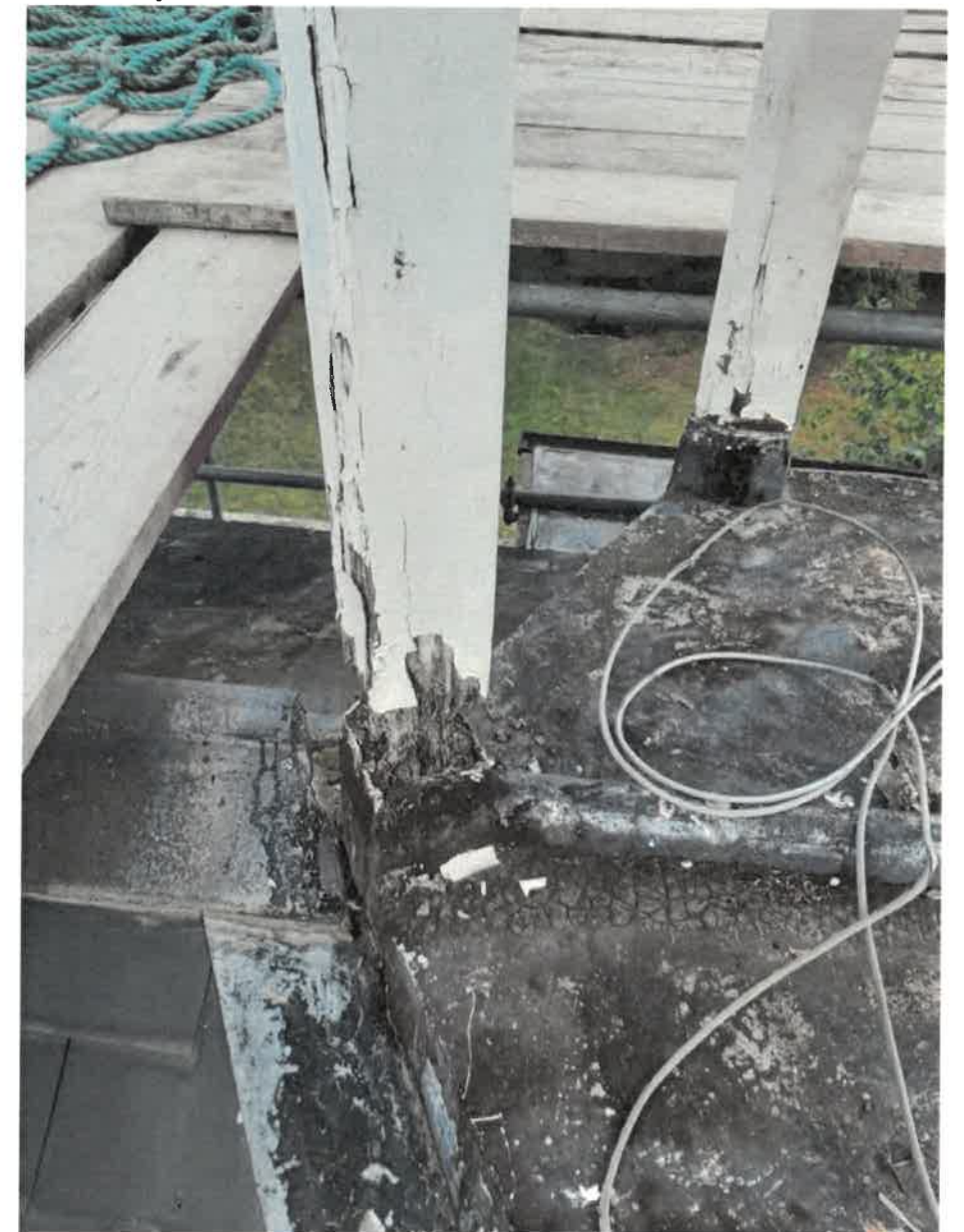
3) Base of cupola post by roof HRFX04.
