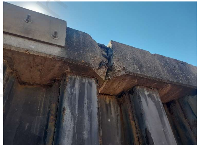
Photo 44 – View of exposed rebar to wall 2 capping beam
