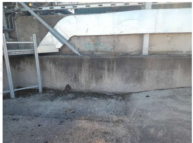
Photo 54 - View of vegetation growth to sealant on wall 5
