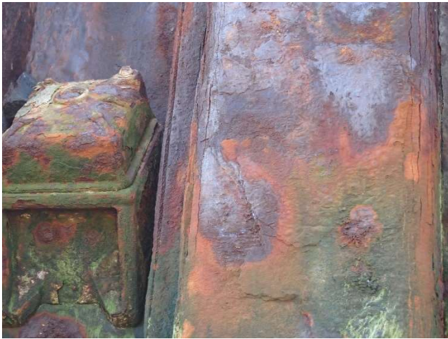
Photo 35 – View of sheet splitting to wall 2
