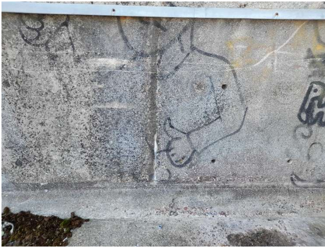
Photo 57 – View of calcite deposits on wall 6
