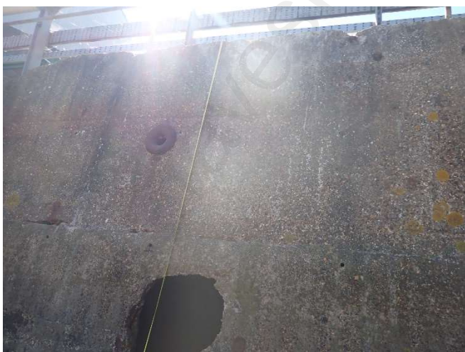
Photo 27 – View of 0.5 m x 0.4 m x 0.19 m void on wall 1
