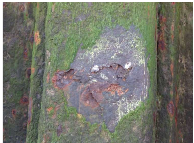
Photo 34 – View of 20 mm delamination to wall 2
