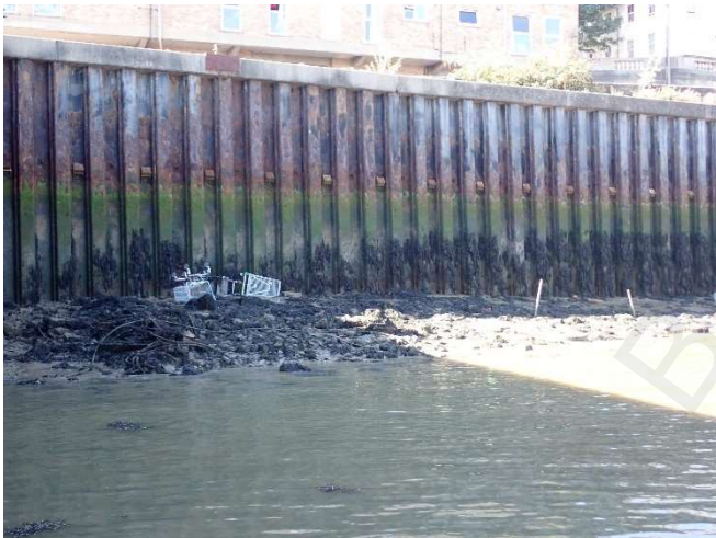
Photo 49 - View of 75% protective coating loss below splash zone
