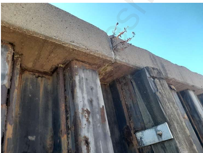
Photo 45 – View of vegetation growth to sealant
