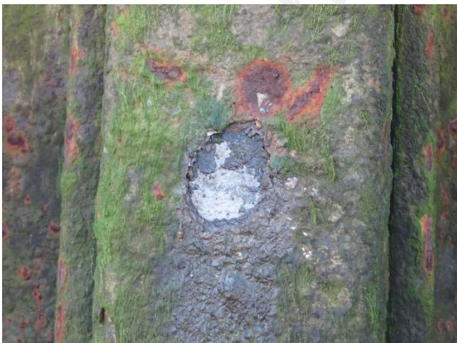
Photo 33 – Typical view of accelerated low water corrosion to wall 2
