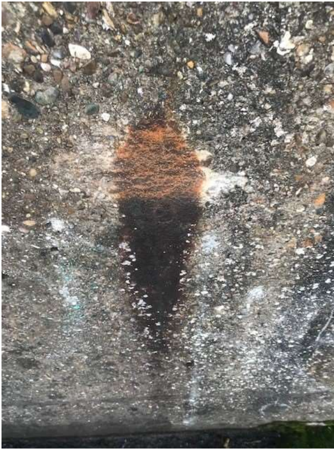
Photo 61 – Stain to wall 5 following wire brushing (by FM Conway).
