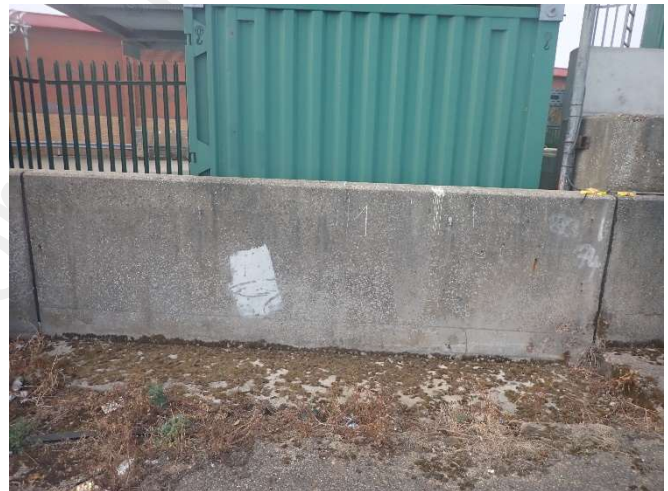
Photo 50 - View of cracking to wall 5
