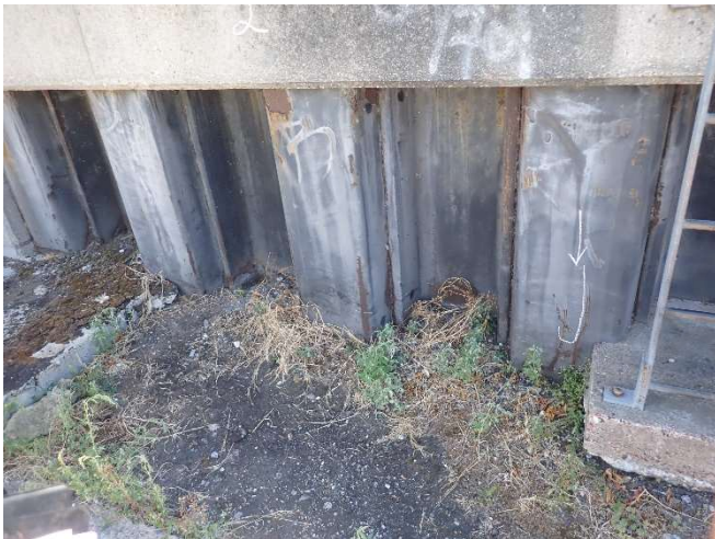
Photo 59 – View of 25% protective coating loss to sheet piling on wall 7
