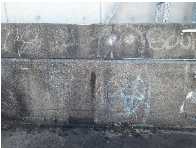
Photo 53 - View of stains and graffiti to wall 5.
