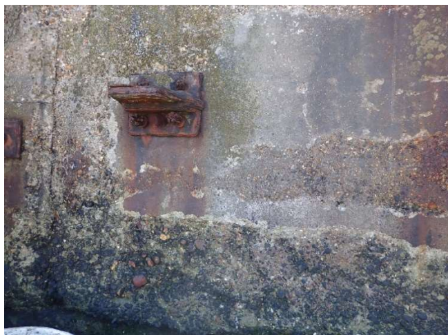
Photo 23- View of honeycombing on wall 1
