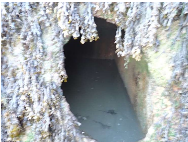
Photo 25 – View of 0.6 x 0.8 x 0.15 m void on wall 1
