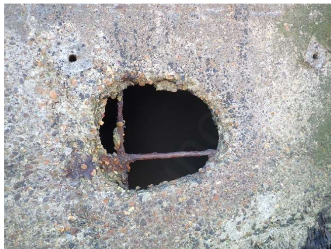
Photo 24 – View of 0.3 x 0.35 x 0.14 m void with rebar visible on wall 1
