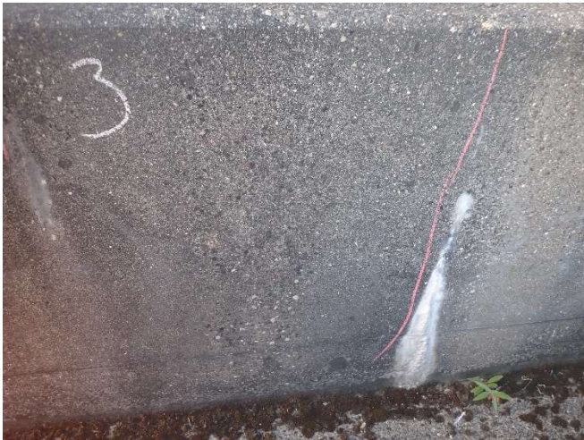
Photo 51 - View of cracking to wall 5
