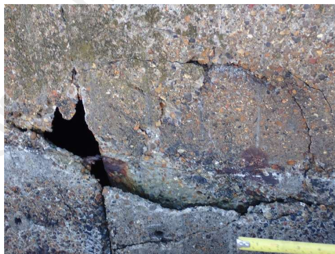
Photo 26 – View of 0.2 x 0.3 x 0.15 m void on wall 1
