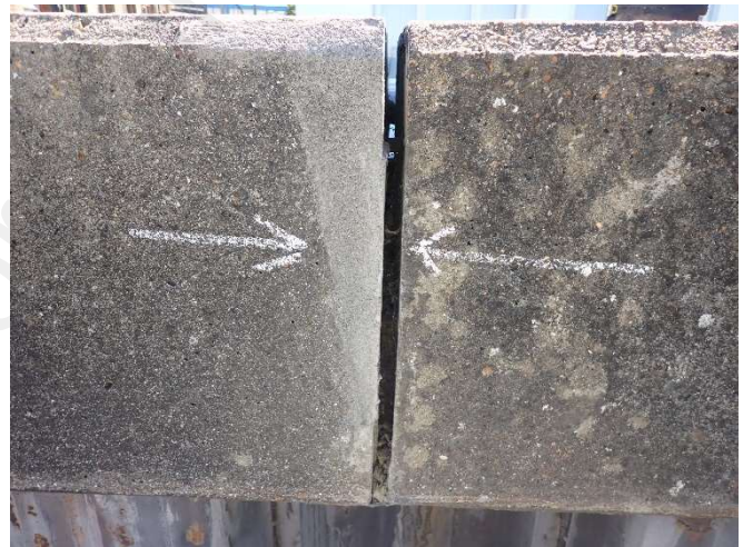
Photo 60 – View of missing sealant between capping beams on wall 7
