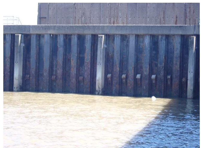
Photo 46 – View of 25% protective coating loss above splash zone to wall 3
