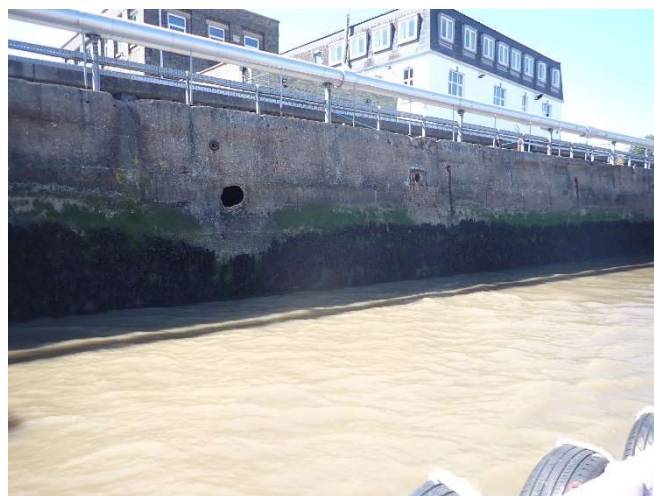
Photo 28 – View of void on wall 1
