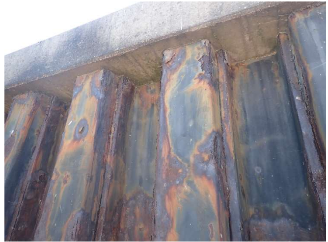
Photo 48 - View of 40% protective coating loss at splash zone on wall 4
