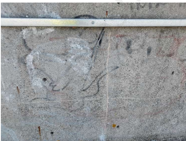
Photo 55 - View of crack on wall 6
