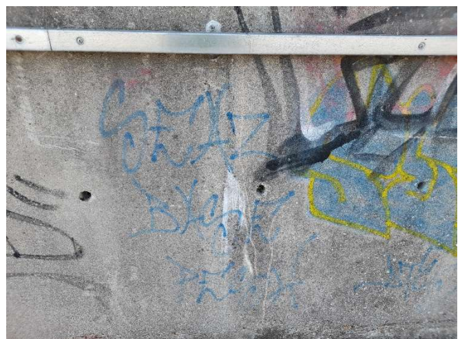
Photo 56 - View of crack on wall 6
