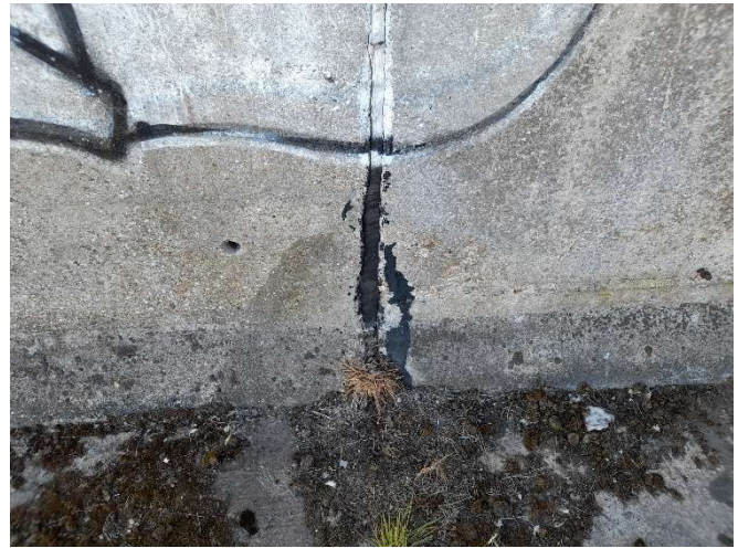
Photo 58 – View of vegetation growth on sealant on wall 6
