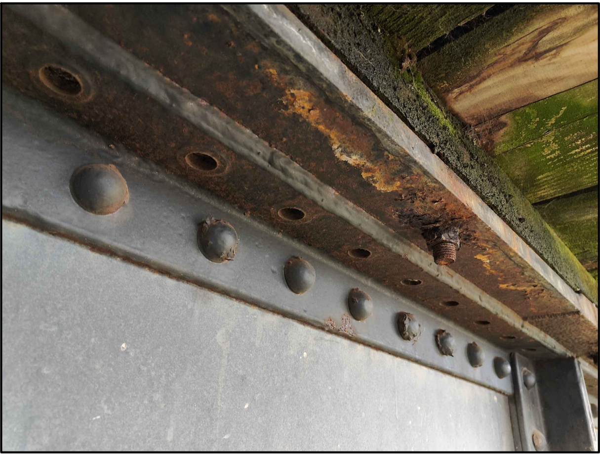
PHOTO 3 - SUPPORTING STEELS WITH TIMBERS IN POOR CONDITION
