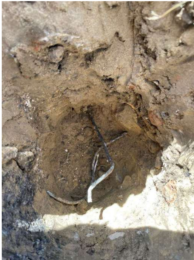
Plate 1: WS01 – refusal on possible reinforced concrete wall of former swimming pool
