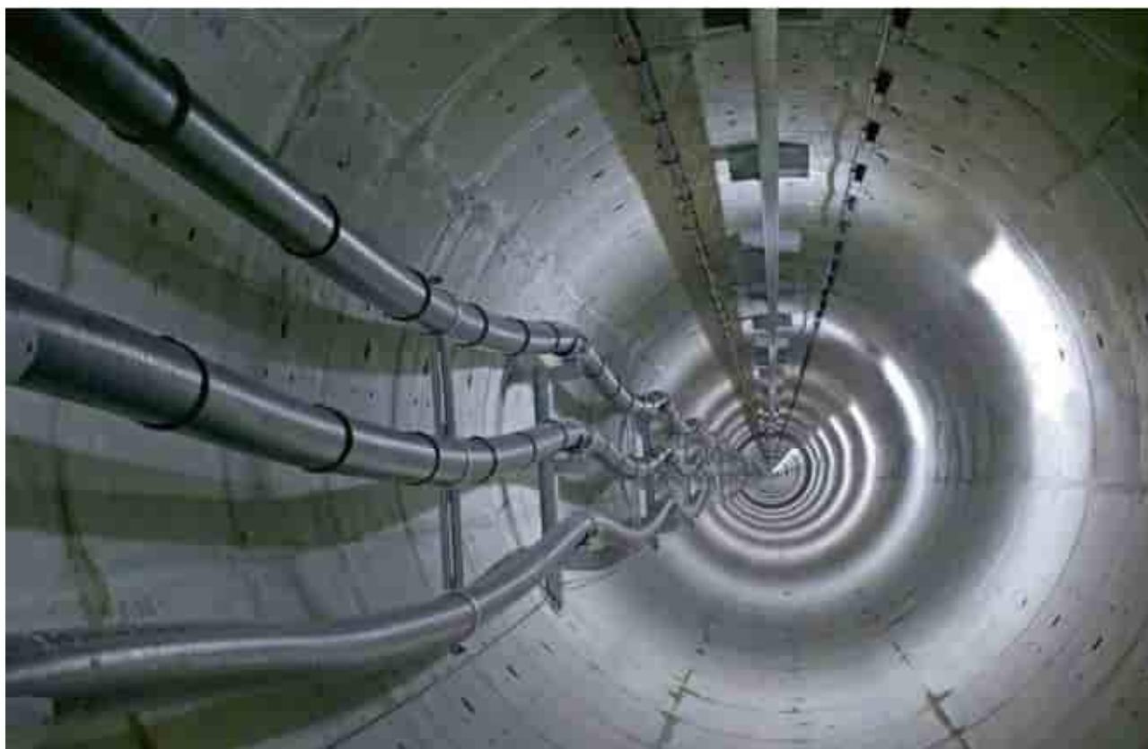
Plate 3-1: Example of XLPE Cables installed in a deep bored tunnel
