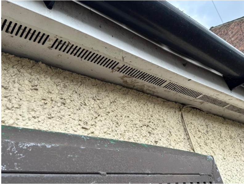
FIGURE 4 – UNDERSIDE OF THE SOFFIT ILLUSTRATING GAPS
