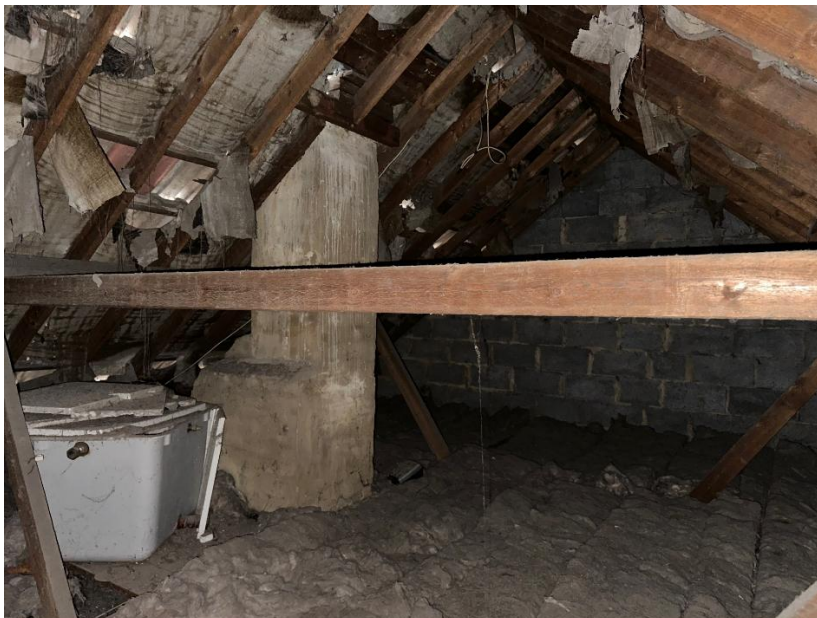
FIGURE 5 – UNDER LINING OF THE ROOF IN POOR CONDITION
