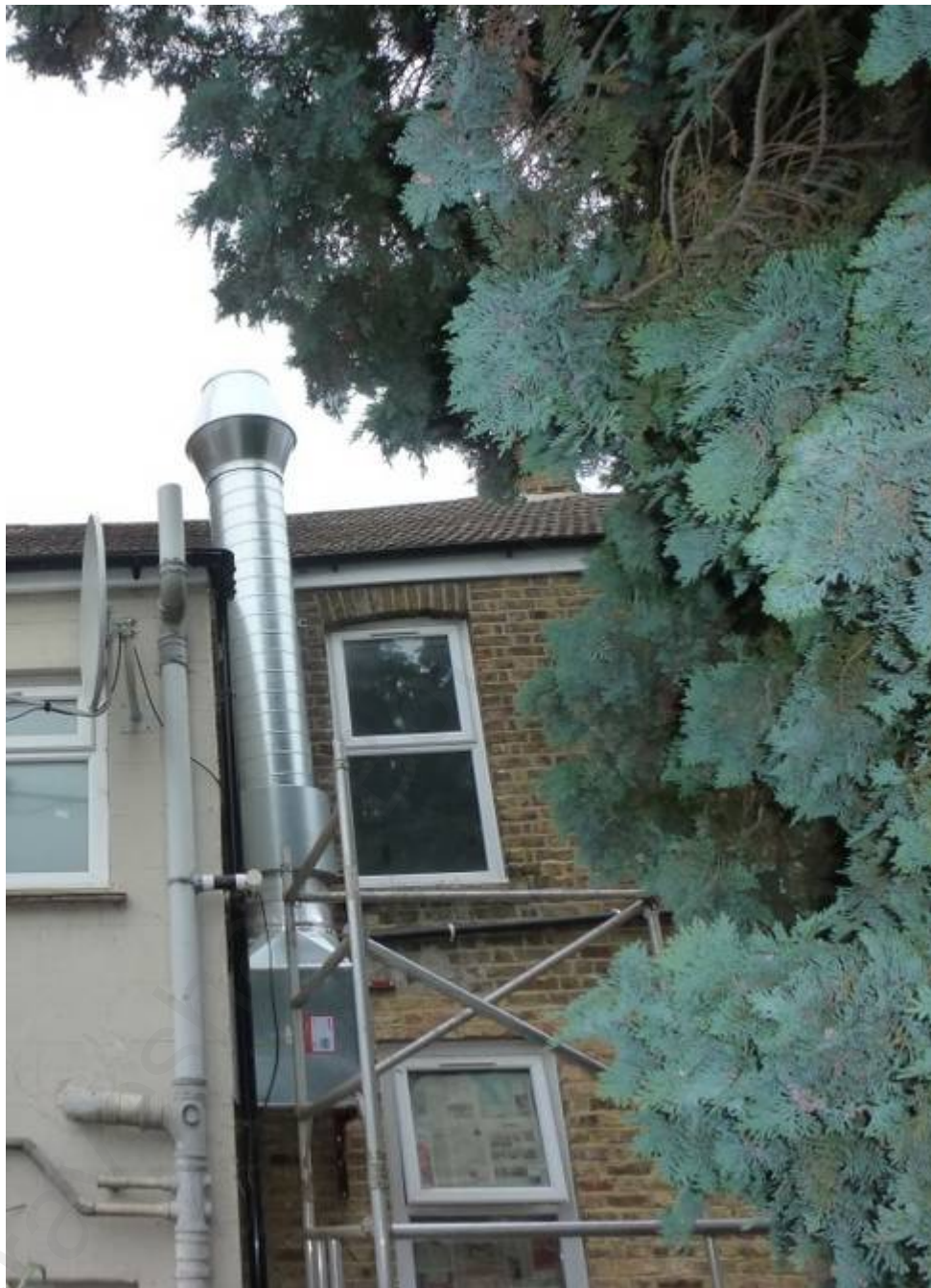
Photo of Extractor installed to rear of the property
