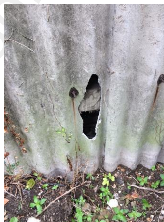
Plate 10- Damaged asbestos cladding along the walls of the barn.
