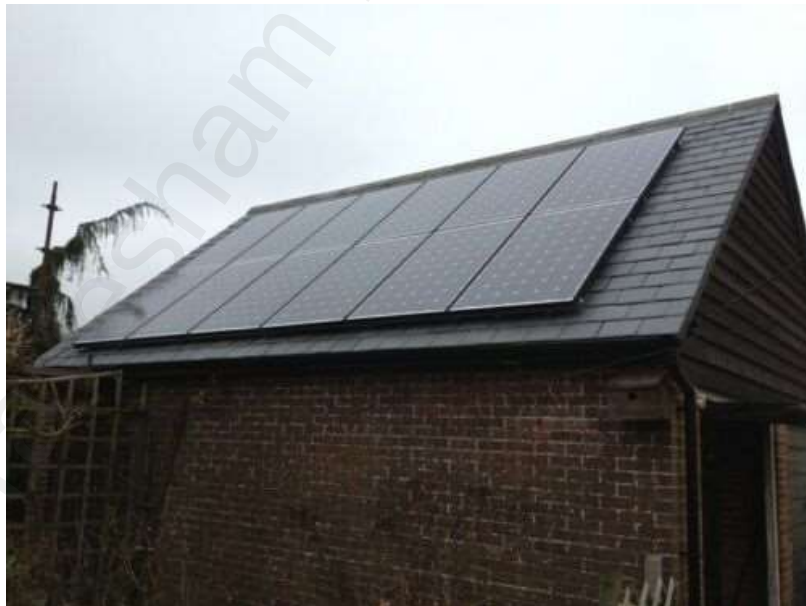
SAMPLE OF SOLAR PANELS
