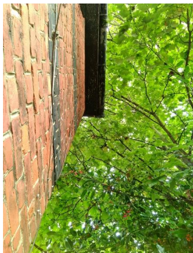
T3 Sycamore (Photo 5) - Foliage smothering building
