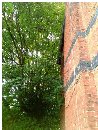
T3 Sycamore (Photo 4) - Foliage smothering building
