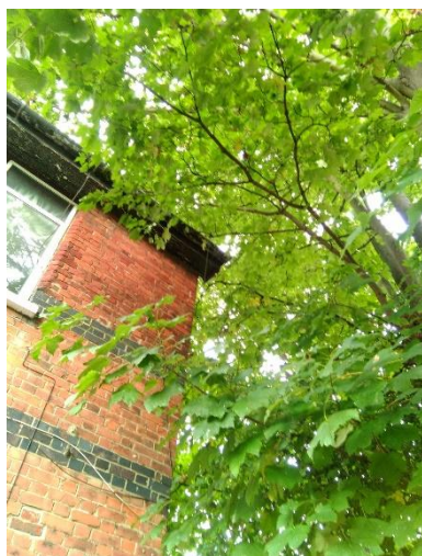
T3 Sycamore (Photo 3) - Foliage smothering building
