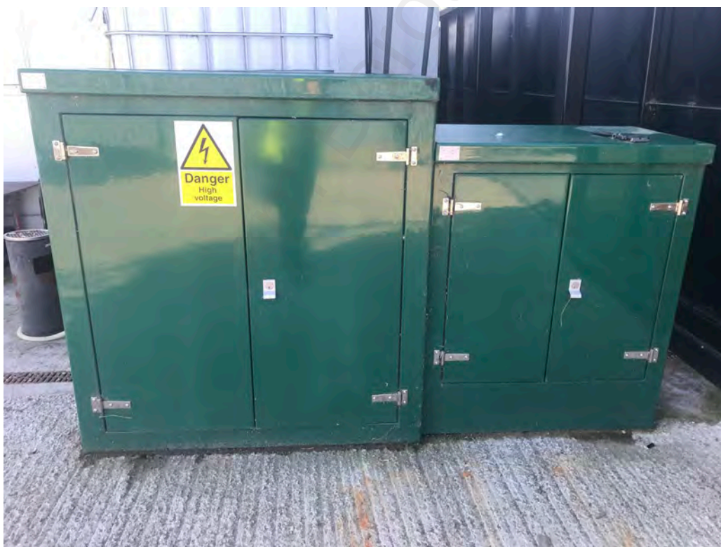
Photographic Plate No. 04: High voltage electricity cabinets in the north western corner of the site.
