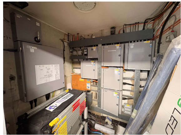
Image 6 – Electrical Cupboard, G.018
