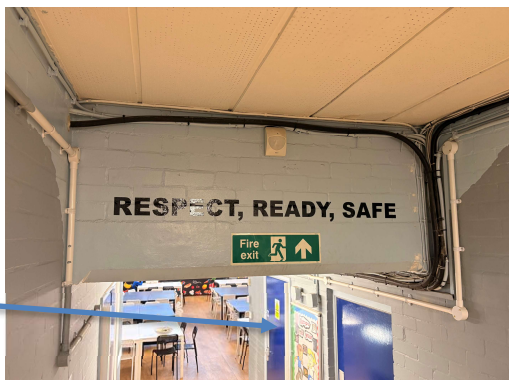
Image 11 – Existing Cable Run from Electrical Cupboard G.018
