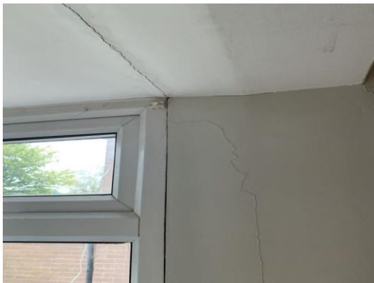
Picture 3: Cracking inside porch
