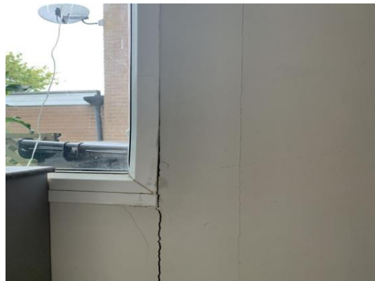
Picture 4: Movement gap in porch
