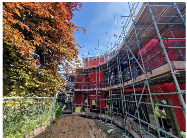
Figure 2. Canopy clearance between T01 and scaffolding.
