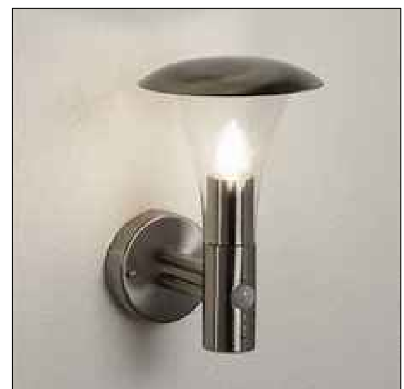
Main front door lights
