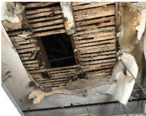
Rot infestation to ceiling
