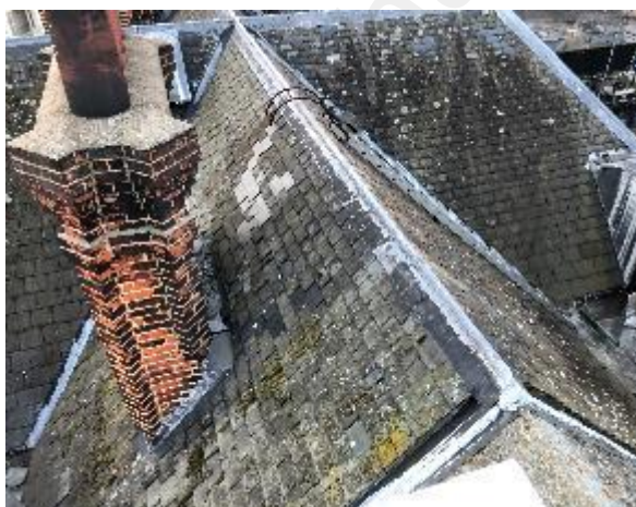
Slipped and broken slates to main roof
