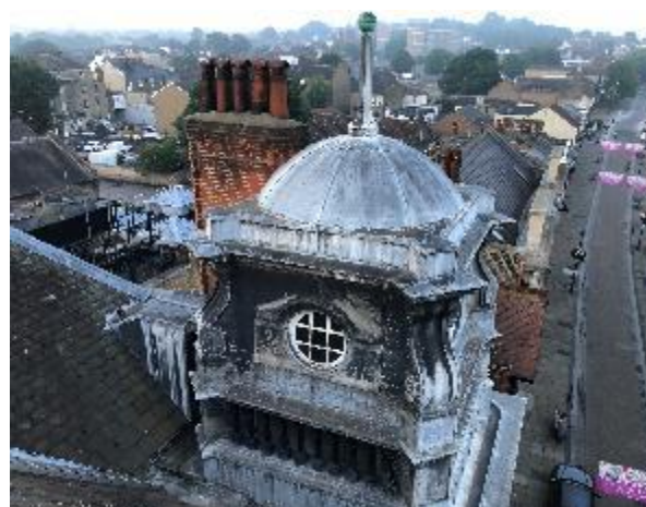
Poorly dressed leadwork to turret
