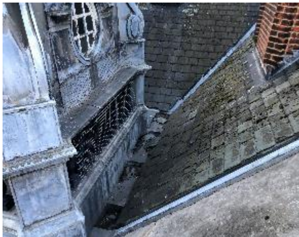
Slipped and broken slates to main roof
