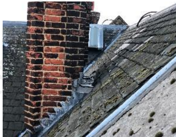
Slipped and broken slates to main roof
