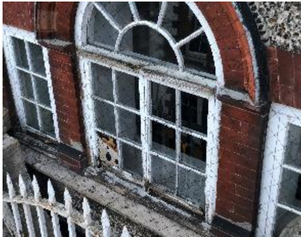
Broken window pane
