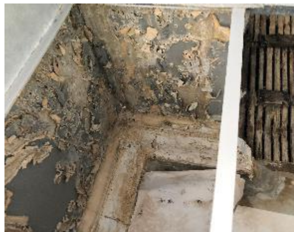
Spalling of plasterwork
