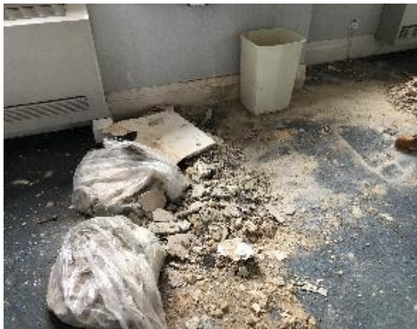
Large amounts of debris from water ingress
