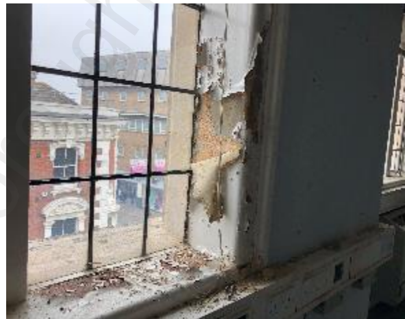
Spalling of plasterwork
