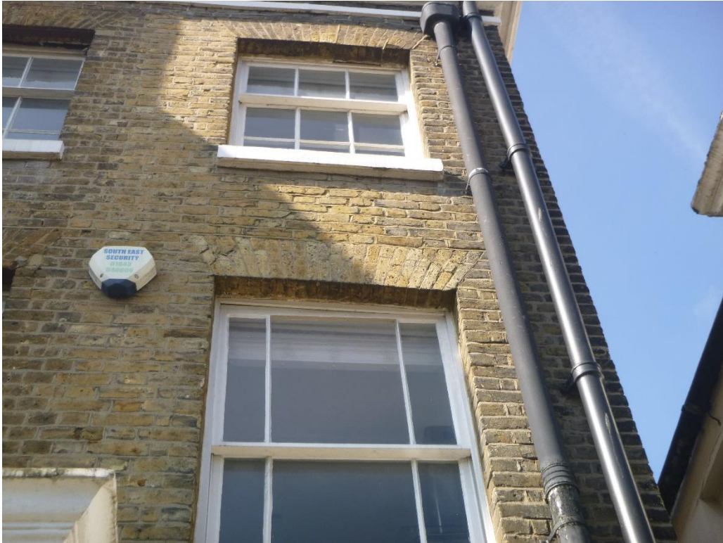
Slipped brick lintel and cracking above on front elevation
