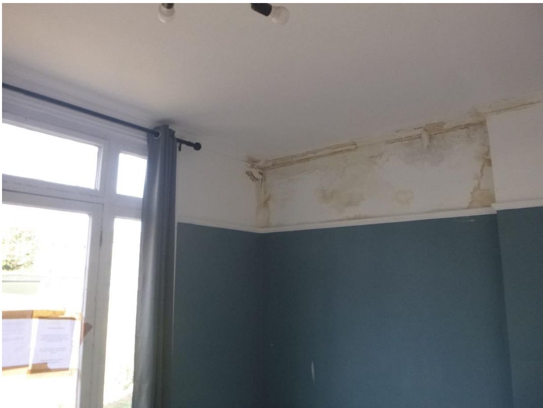
Damp ingress at top of flank wall
