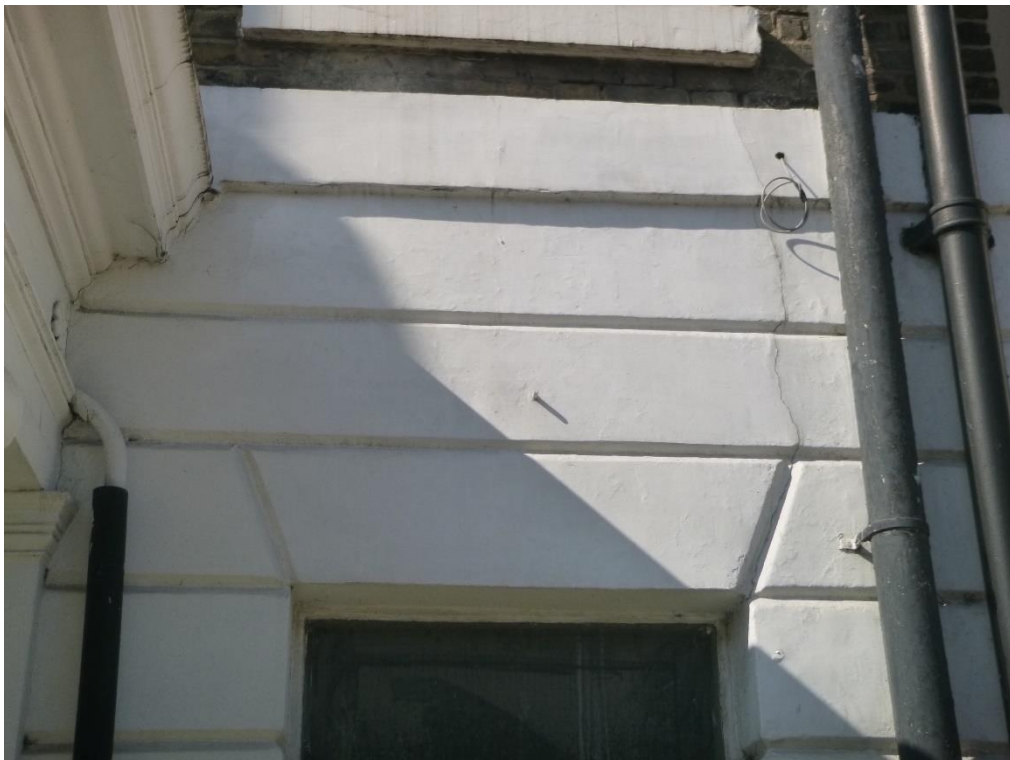
Cracking to stonework at first floor level on right hand side of front elevation
