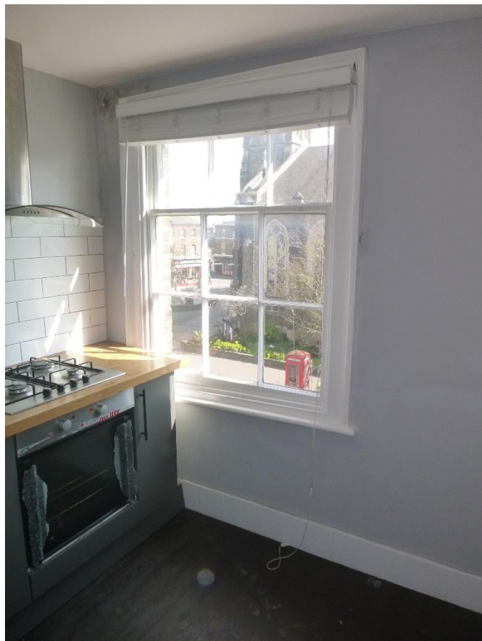
Historic distortion of window cill adjacent to flank wall
