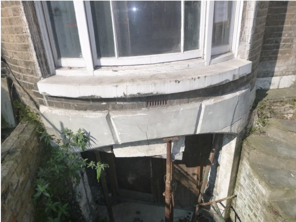
Cracking to front bay at ground floor level (Frame removed and temporary props under)
