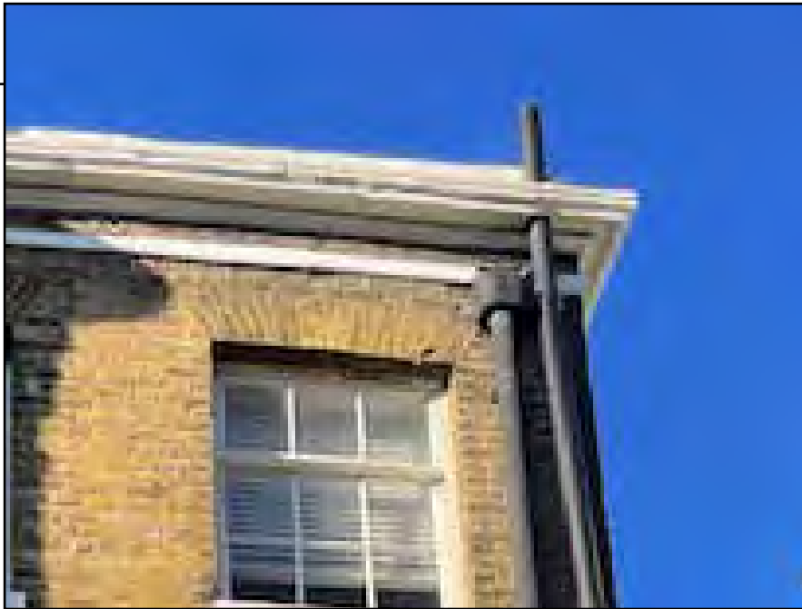
Front elevation - there is evidence of suspected rainwater goods debris blockages Resulting in brickwork failure with water ingress into the brick mortar
