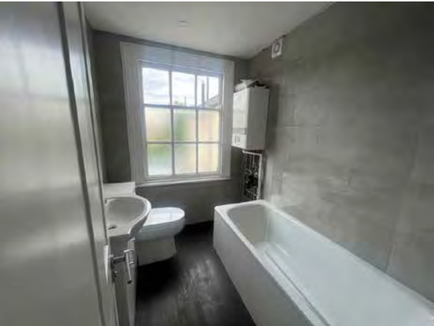
View A - bathroom interior rear looking west toward rear sash opaque glass window. Noteworthy - window and frame in tack.
