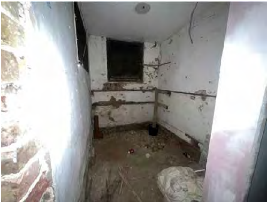
View A - No. 195 existing basement smaller light well window and interior side wall window- evidence of aborted works
