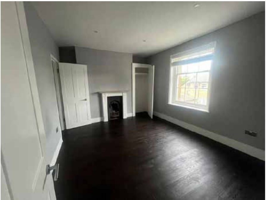
View C - No. 195 second floor rear bedroom looking south toward fireplace Noteworthy - fireplace, mantel, grate, window, sill, cupboard still in tack Evidence of replacement door and modern electrical fittings
