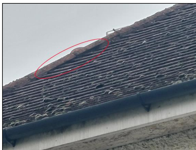
Photograph 2. Missing pugging from below the ridge tile on the left side of the rear elevation as highlighted in red.
