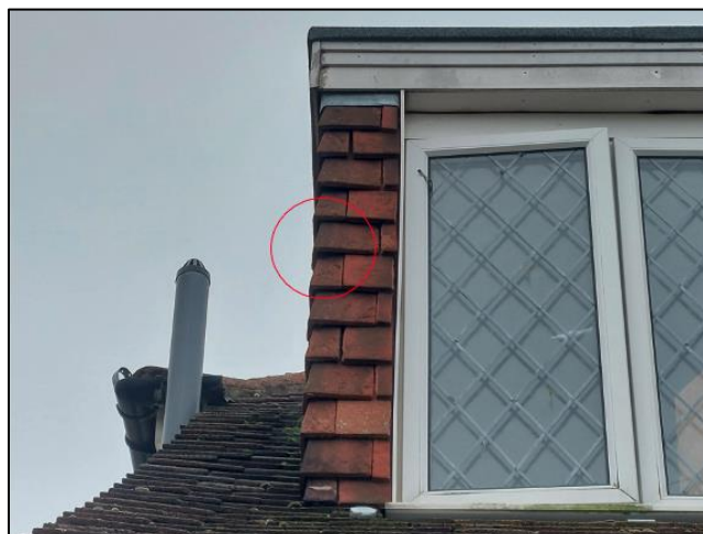
Photograph 6. Gaps present on the hanging tiles of the dormer window on the front elevation as highlighted in red.
