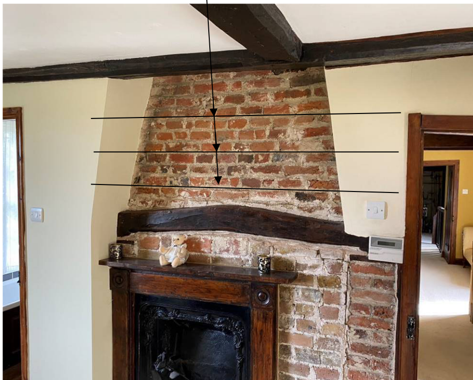
Plate 5 – Slight Cracking Above First Floor Fireplace Bressummer and Loose Infill Masonry
