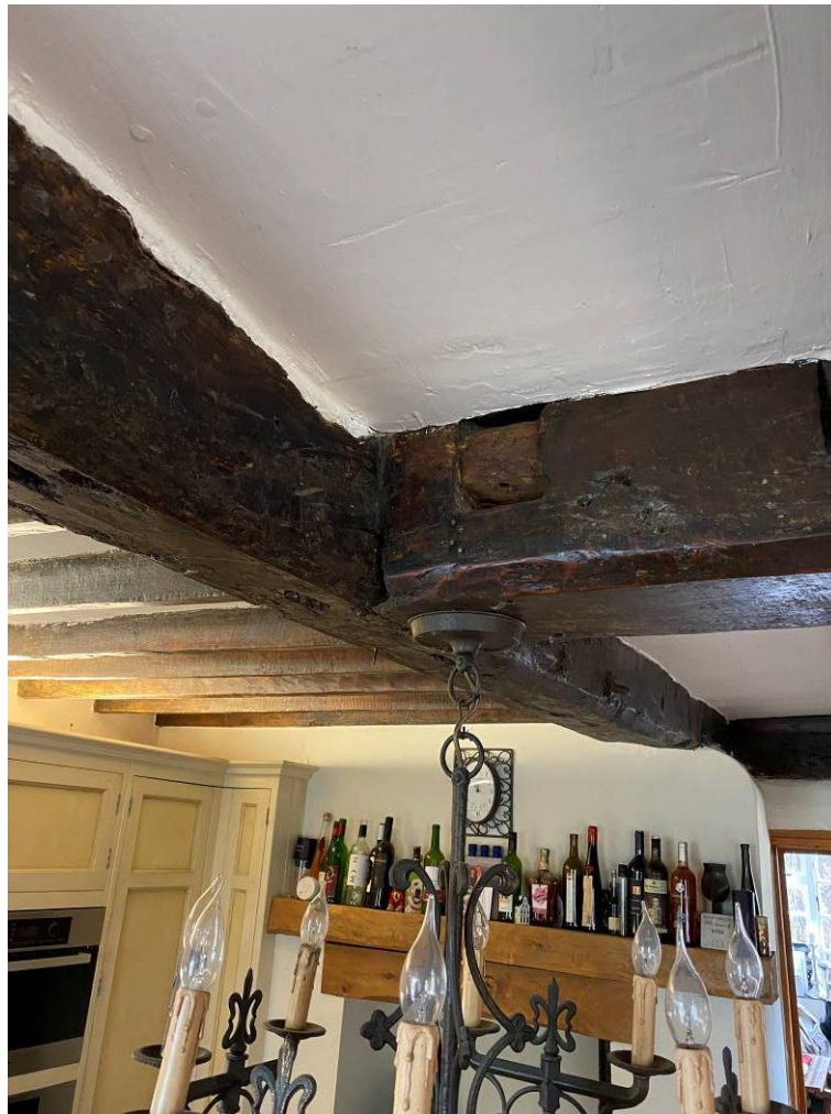
Plate 3 – Slight Opening of Joint Between Kitchen Beams
