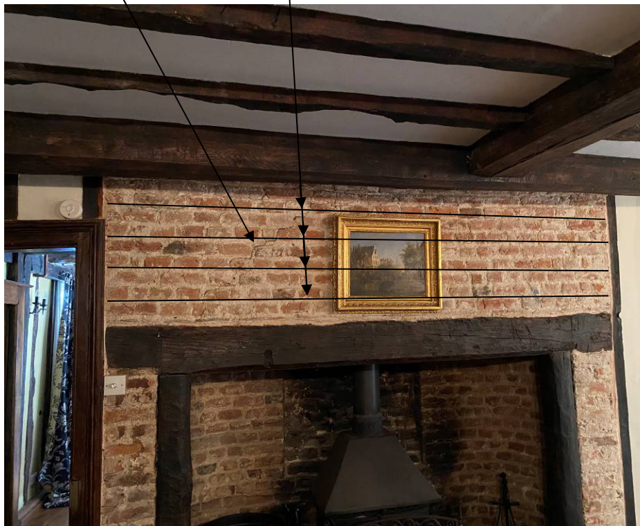
Plate 4 – Cracking Above Lounge Fireplace Bressummer
