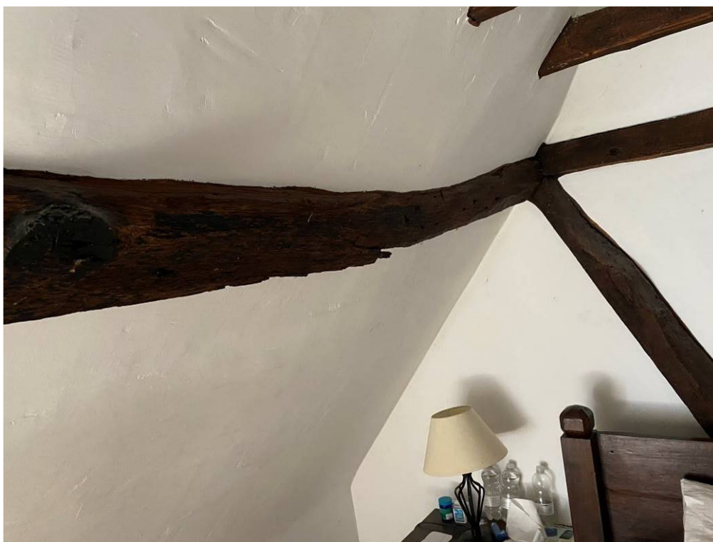
Plate 7 – Fracture to Second Floor Loft Room Purlin
