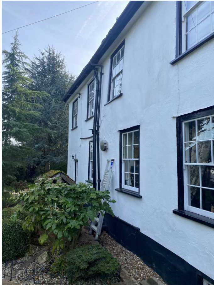
Plate 1 – Bulge to North Wall
