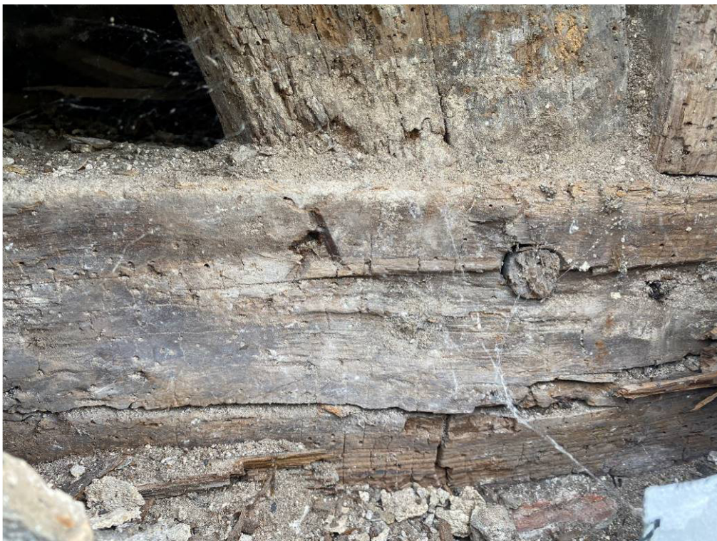
Plate 2 – Slight Fracture to First Floor Soleplate
