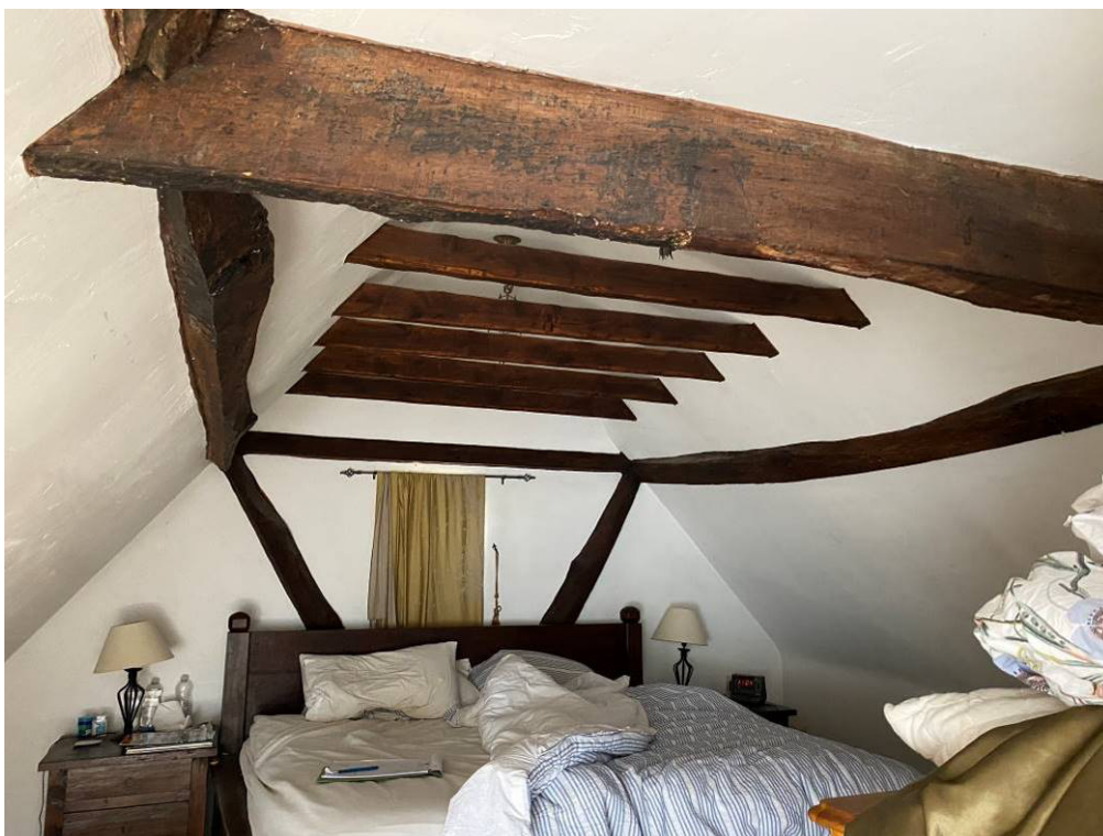
Plate 6 – Bowed Purlin to Second Floor Loft Room
