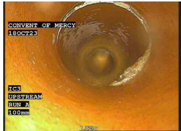
2, 00:00:28, 1.82 m Attached deposits, encrustation at joint from 03 o'clock to 06 o'clock, 5% cross-sectional area loss
