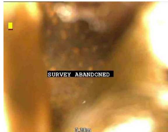
2, 00:00:12, 0.30 m Survey abandoned, Unable to continue
