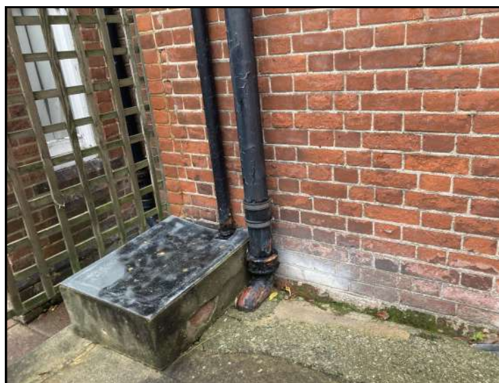
SVP 2. UNABLE TO CCTV
