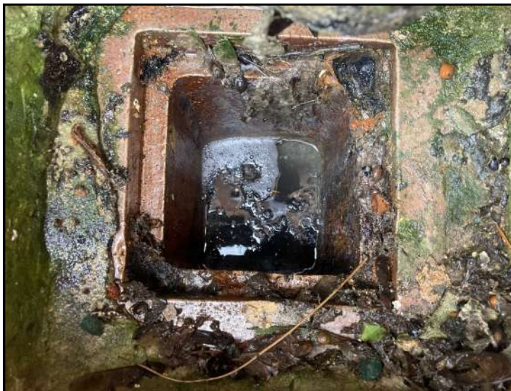
COMBINED GULLY 1. TRAPPED - NO CCTV
