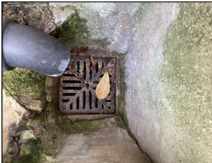
FOUL GULLY 1. TRAPPED - NO CCTV
