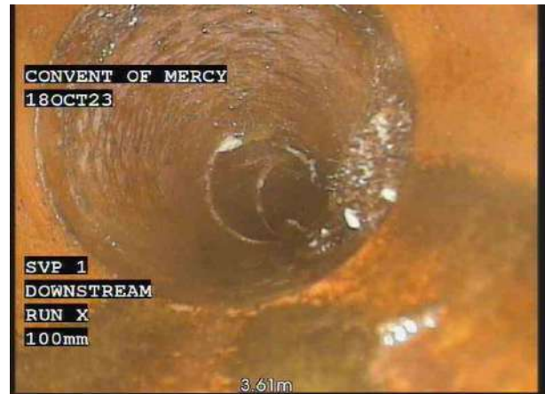
2, 00:01:28, 3.61 m Roots, mass at joint, 5% cross-sectional area loss
