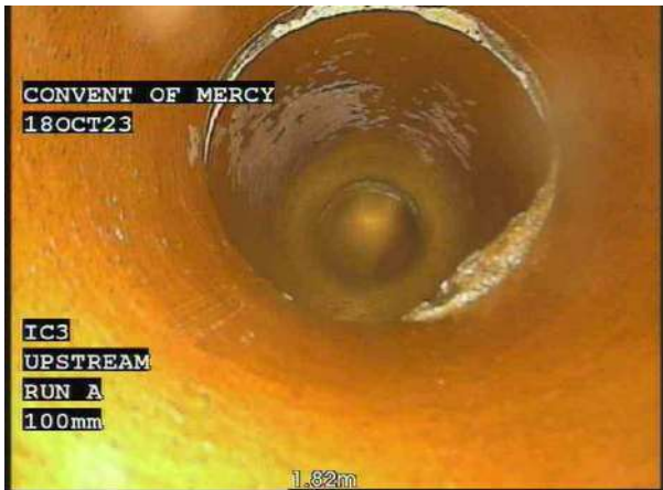
1, 00:00:20, 1.82 m Crack, circumferential at joint from 09 o'clock to 02 o'clock
