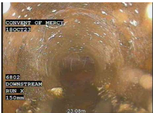
5, 00:03:46, 23.08 m Roots, mass at joint, 5% cross-sectional area loss
