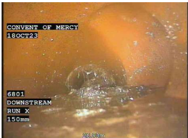
3, 00:03:59, 28.93 m Settled deposits, hard or compacted, 20% cross-sectional area loss
