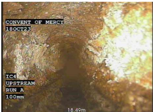
3, 00:02:47, 18.49 m Attached deposits, encrustation from 07 o'clock to 05 o'clock, 5% cross-sectional area loss, start
