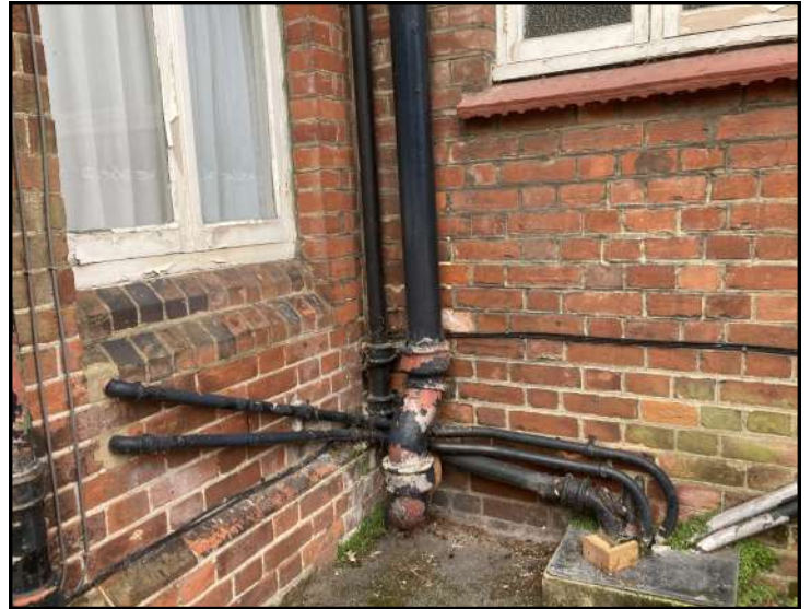
LOCATION OF VENT PIPE 1
