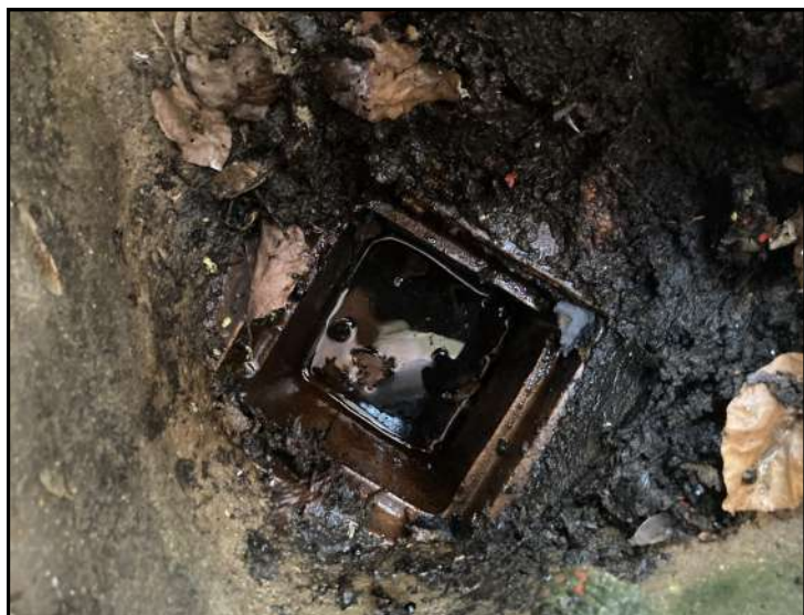
COMBINED GULLY 2. TRAPPED - NO CCTV
