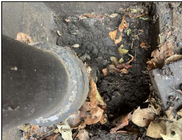
RWP + GULLY 1. DEBRIS FILLED
