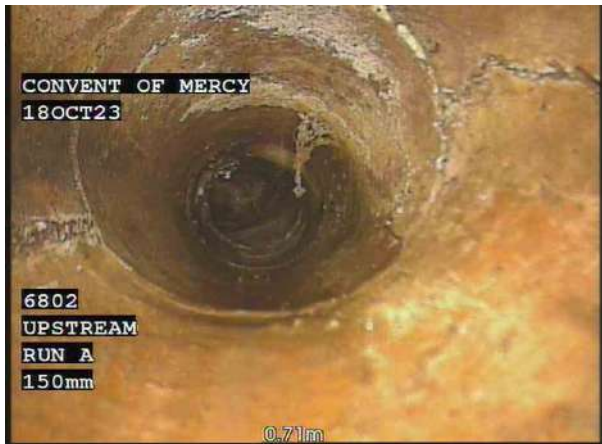
1, 00:00:16, 0.71 m Fracture, longitudinal at joint at 3 o'clock
