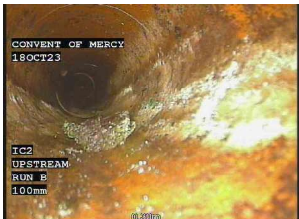
1, 00:00:08, 0.30 m Crack, circumferential from 10 o'clock to 02 o'clock
