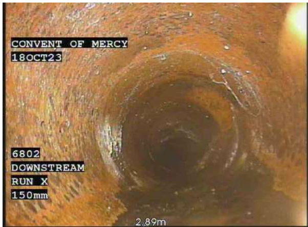
1, 00:00:29, 2.89 m Attached deposits, encrustation from 05 o'clock to 07 o'clock, 5% cross-sectional area loss
