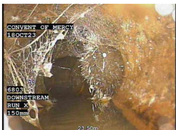
3, 00:02:20, 23.50 m Roots, mass, 10% cross-sectional area loss
