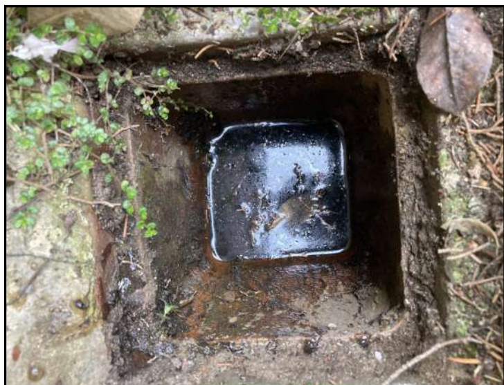
GULLY 1. TRAPPED - NO CCTV
