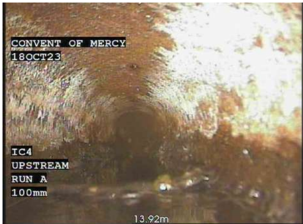
1, 00:01:49, 13.92 m Settled deposits, hard or compacted, 5% cross-sectional area loss
