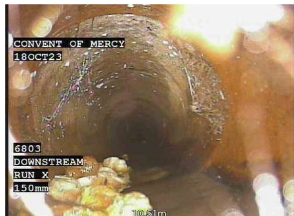
2, 00:01:00, 10.51 m Roots, fine at joint
