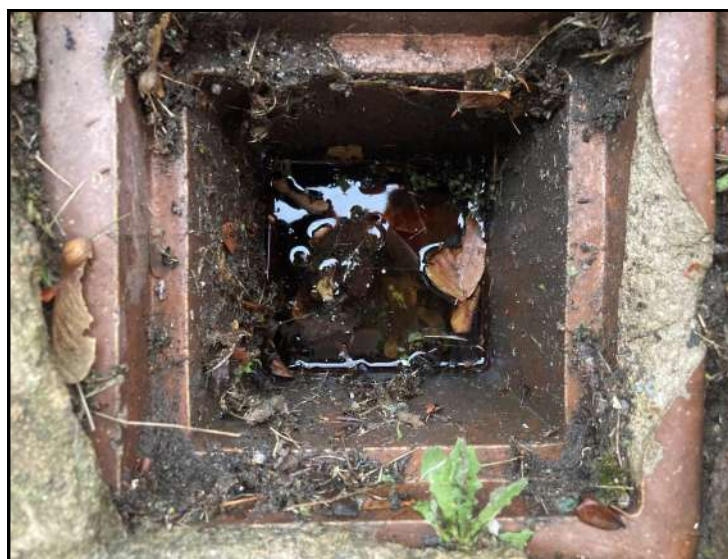
GULLY 3. TRAPPED - NO CCTV
