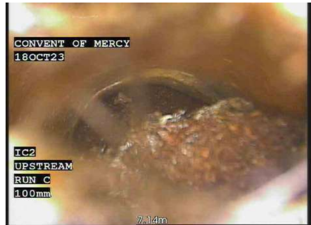
2, 00:01:44, 7.14 m Settled deposits, hard or compacted, 90% cross-sectional area loss
