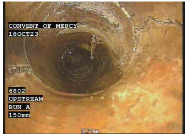
2, 00:00:23, 0.71 m Fracture, longitudinal at joint at 8 o'clock
