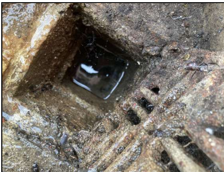
FOUL GULLY 2. TRAPPED - NO CCTV
