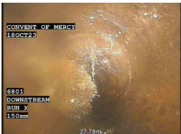
5, 00:05:36, 37.78 m Roots, mass at joint, 30% cross-sectional area loss
