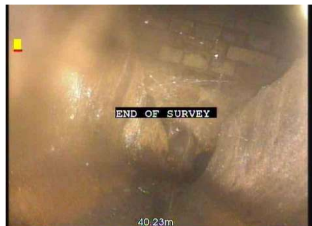
6, 00:06:09, 40.23 m Finish node, manhole, reference: 6804, Unable to lift - buried / covered over
