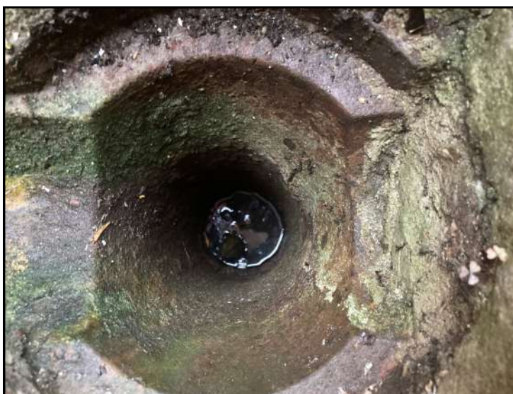
FOUL GULLY 5. TRAPPED - NO CCTV
