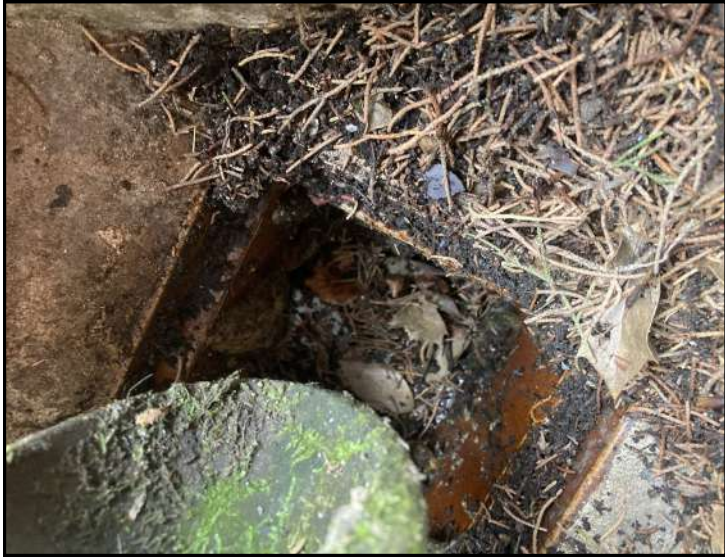
RWP + GULLY 3. TRAPPED - NO CCTV
