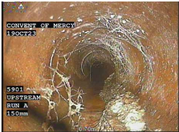
1, 00:00:26, 0.70 m Roots, mass at joint, 5% cross-sectional area loss
