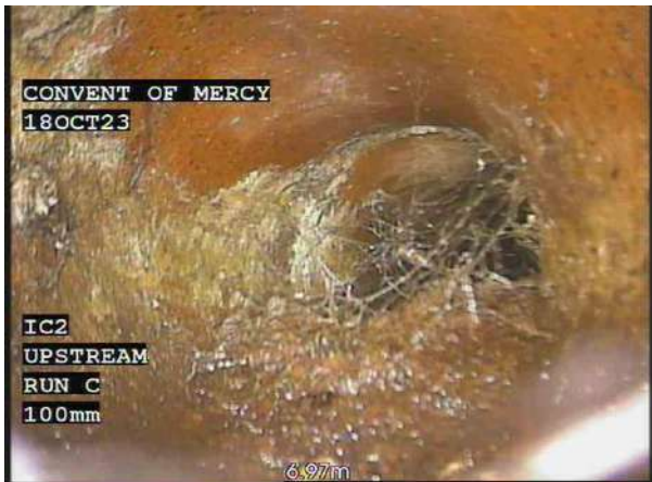
1, 00:01:20, 6.97 m Settled deposits, hard or compacted, 20% cross-sectional area loss
