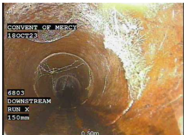
1, 00:00:05, 0.50 m Roots, fine at joint
