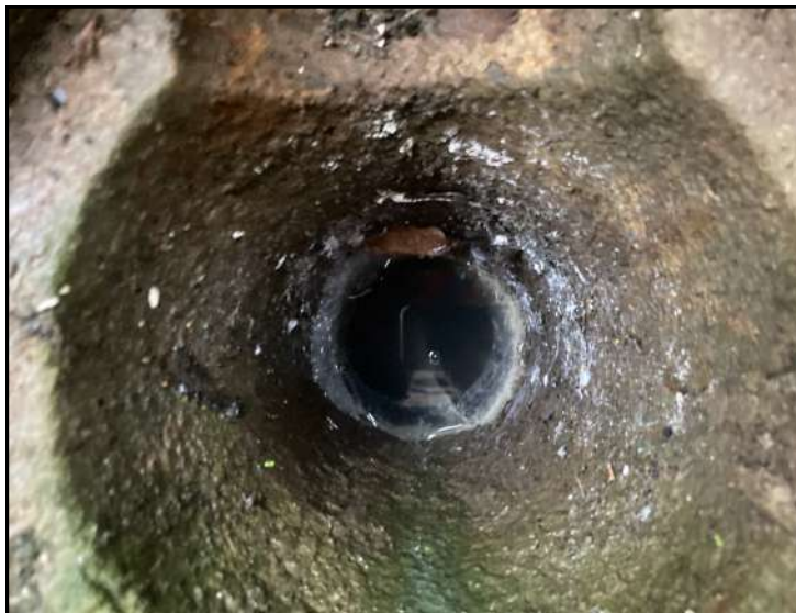
FOUL GULLY 4. TRAPPED - NO CCTV
