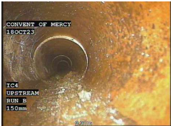
1, 00:00:42, 3.31 m Settled deposits, hard or compacted, 5% cross-sectional area loss, start
