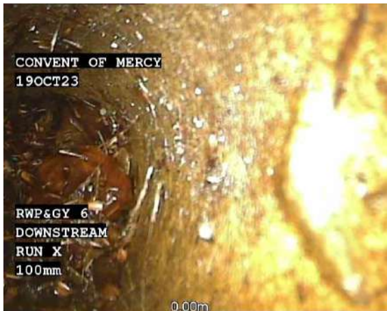
1, 00:00:02, 0.00 m Settled deposits, hard or compacted, 95% cross-sectional area loss
