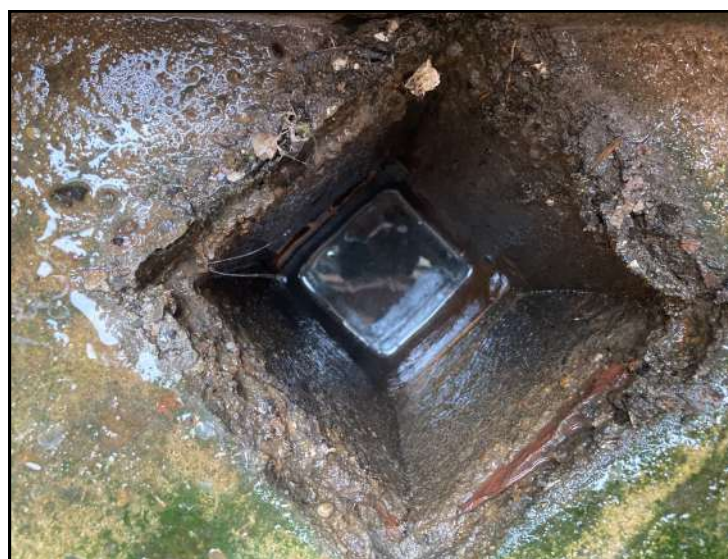
COMBINED GULLY 3. TRAPPED - NO CCTV
