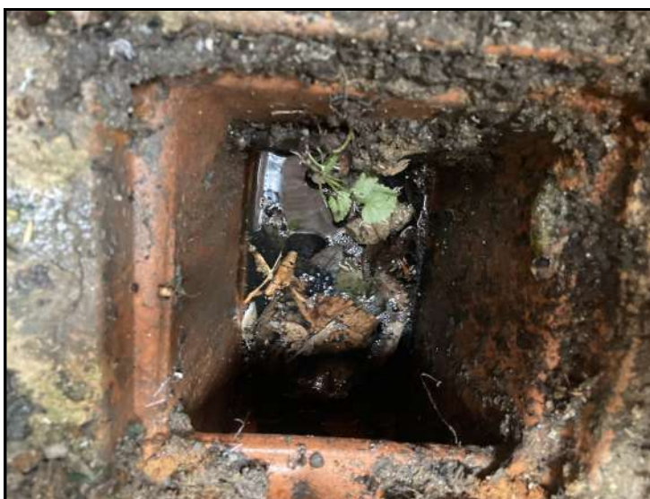
RWP + GULLY 5. TRAPPED - NO CCTV
