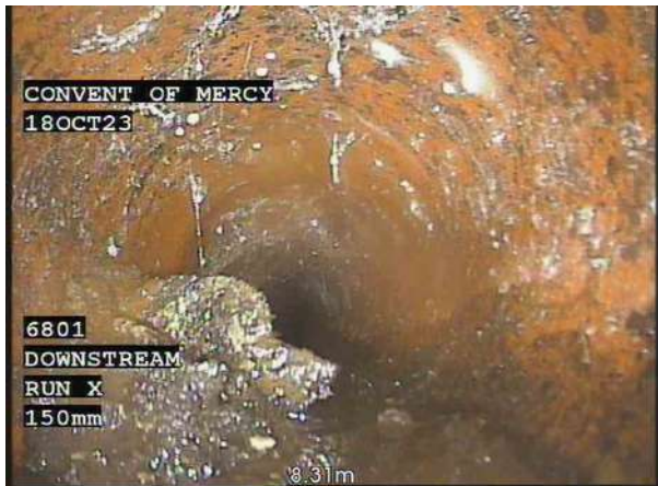
1, 00:00:46, 8.31 m Settled deposits, hard or compacted, 10% cross-sectional area loss
