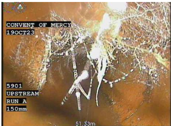
3, 00:07:16, 51.33 m Roots, mass at joint, 5% cross-sectional area loss
