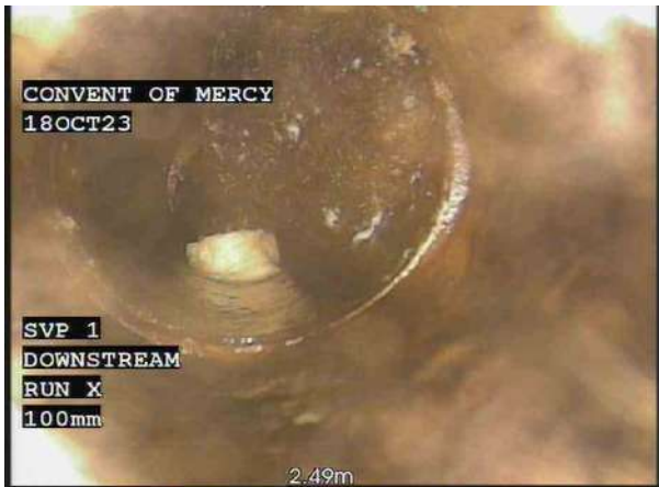
1, 00:00:54, 2.49 m Roots, mass at joint, 25% cross-sectional area loss
