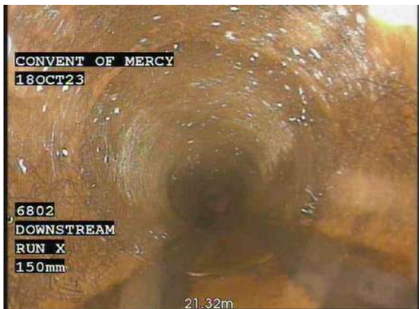
3, 00:02:58, 21.32 m Roots, fine at joint
