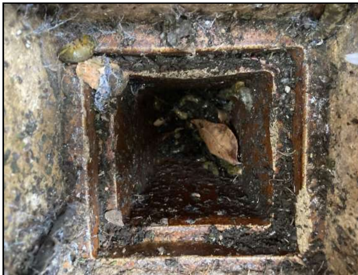
RWP + GULLY 4. TRAPPED - NO CCTV
