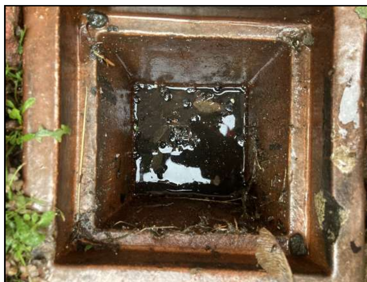
GULLY 2. TRAPPED - NO CCTV
