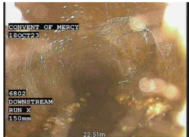
4, 00:03:27, 22.51 m Settled deposits, hard or compacted, 5% cross-sectional area loss
