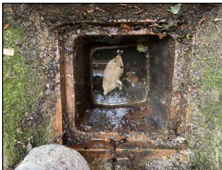
COMBINED GULLY 4. TRAPPED - NO CCTV
