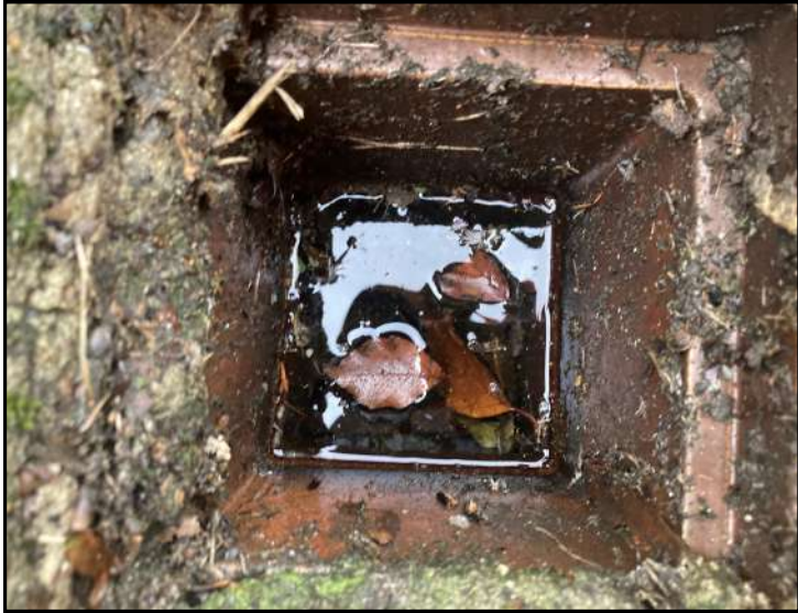
GULLY 4. TRAPPED - NO CCTV
