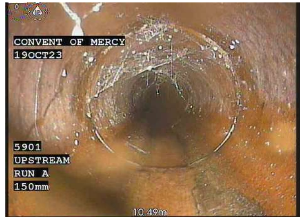
2, 00:01:45, 10.49 m Attached deposits, encrustation from 05 o'clock to 07 o'clock, 5% cross-sectional area loss, start
