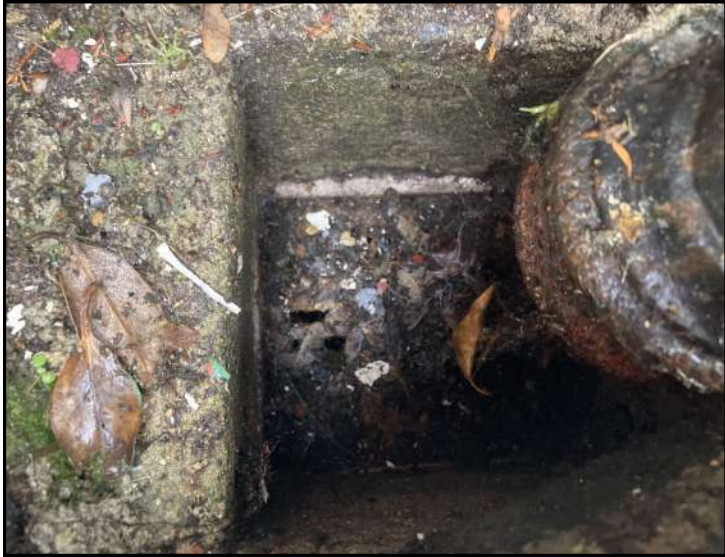
FOUL GULLY 3. TRAPPED - NO CCTV
