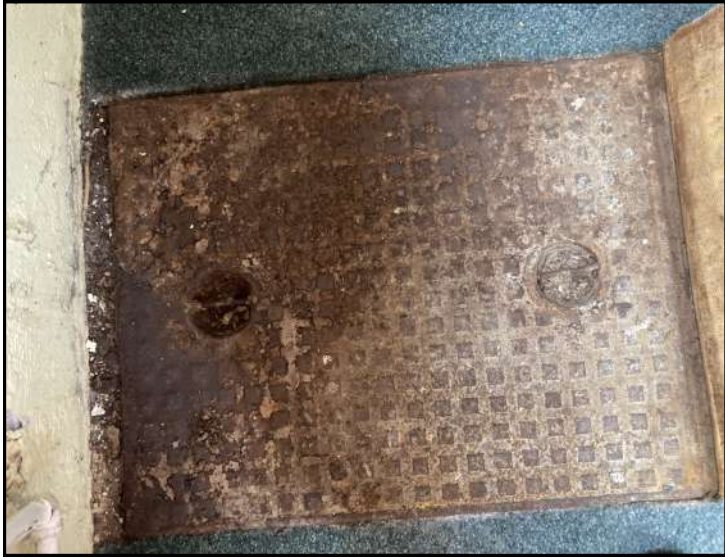
IC7. INTERNAL. UNABLE TO LIFT - COVER SEIZED
