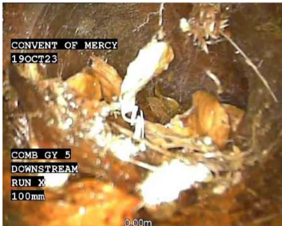
1, 00:00:00, 0.00 m Settled deposits, hard or compacted, 10% cross-sectional area loss, start
