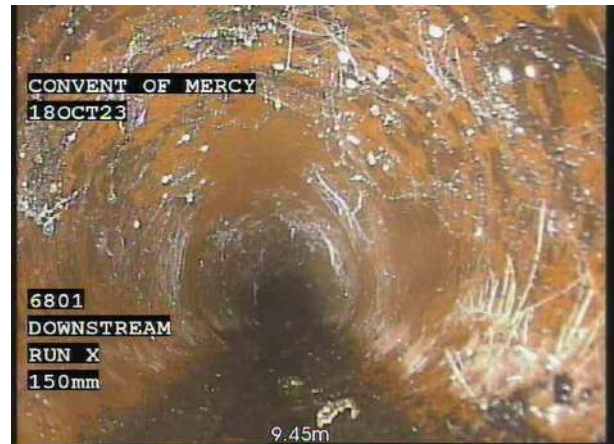
2, 00:01:07, 9.45 m Settled deposits, hard or compacted, 5% cross-sectional area loss, start
