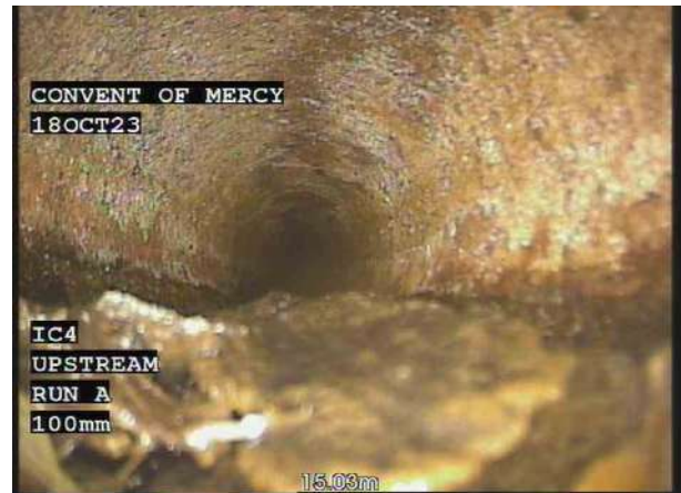
2, 00:02:12, 15.03 m Settled deposits, hard or compacted, 10% cross-sectional area loss
